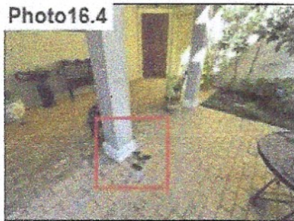
Substrate Damage / Assess & Repair
