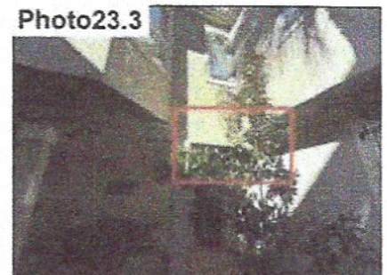
Substrate Damage / Assess, Repair and Install Proper Relief
