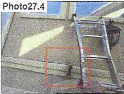
Substrate Damage / Assess & Repair
