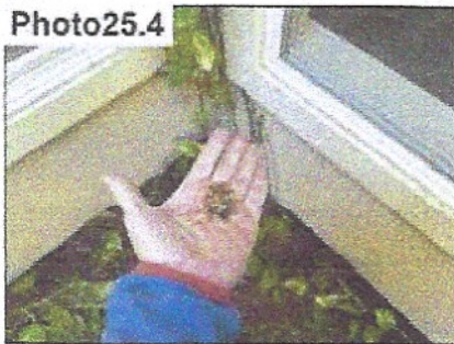
Wood Rot at Bottom Wall/ Repair
