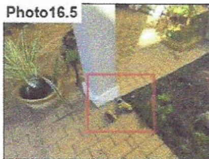
Substrate Damage / Assess & Repair
