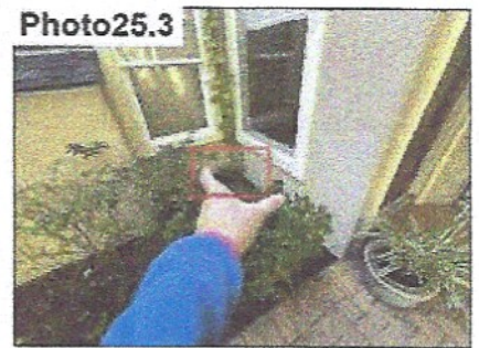
Wood Rot at Bottom Wall/ Repair
