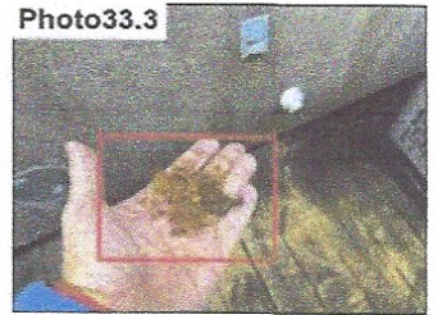
Substrate Damage / Assess & Repair
