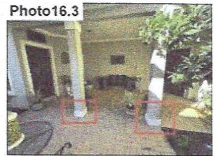
Substrate Damage / Assess & Repair
