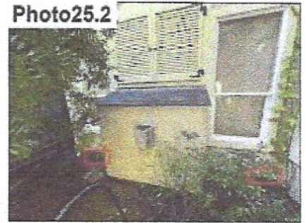
Wood Rot at Bottom Wall/ Repair
