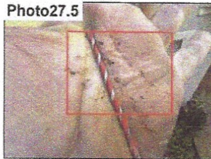
Substrate Damage / Assess & Repair
