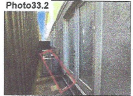
Substrate Damage / Assess & Repair
