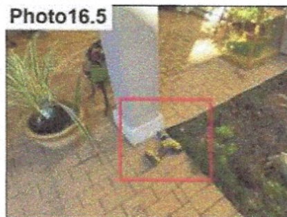
Substrate Damage / Assess & Repair
