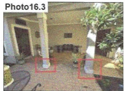
Substrate Damage / Assess & Repair
