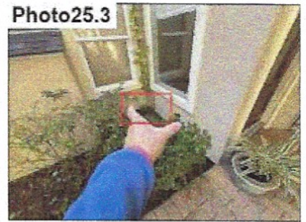
Wood Rot at Bottom Wall/ Repair
