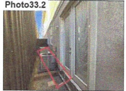
Substrate Damage / Assess & Repair
