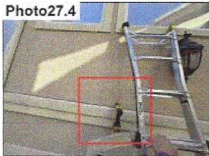
Substrate Damage / Assess & Repair
