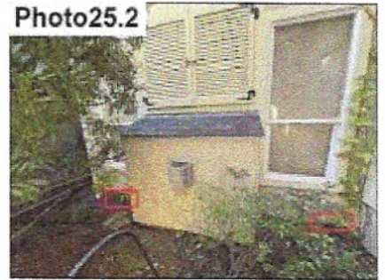
Wood Rot at Bottom Wall/ Repair
