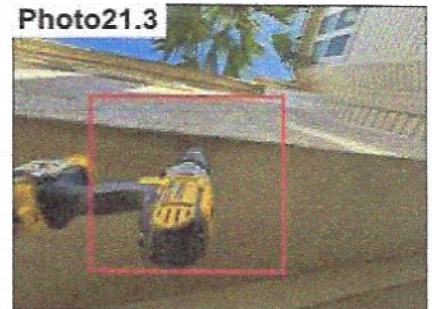
Photo21.3 Substrate Damage / Assess, Repair and Install Proper Relief
