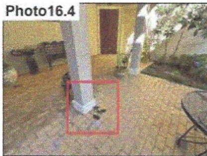
Substrate Damage / Assess & Repair
