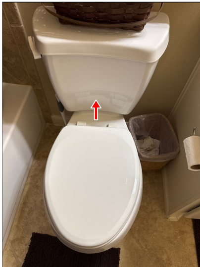
A. Item 2 Commode tank is loose at the bowl at hall bath
