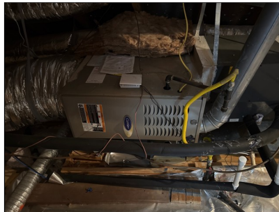
A. Item 2 The heating unit appeared to operate normally using the standard controls at master bedroom system
