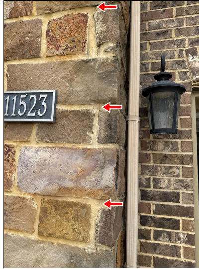
F. Item 9 Observed cracks in stone veneer at right side of entry
