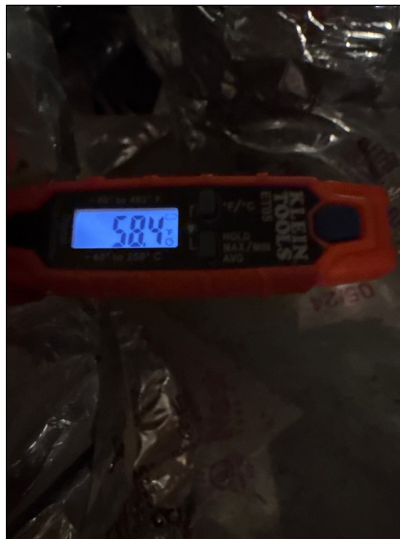
B. Item 2 Supply Side
