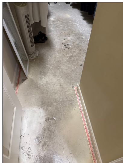
G. Item 1 Observed missing floor covering at master closet
