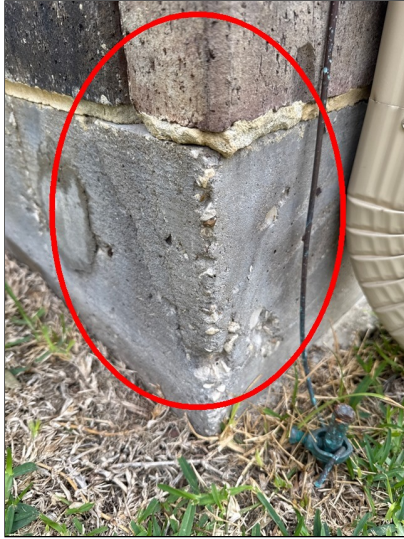
A. Item 2 Common corner crack observed at left rear corner of home
