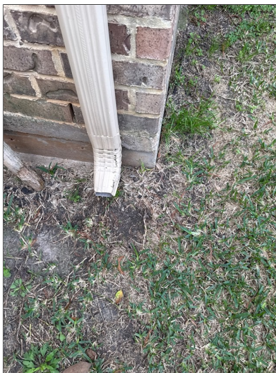
B. Item 2 Splash block or downspout extensions are absent at right rear corner of garage
