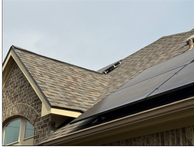
C. Item 8 This roof covering is probably around 5-7 years old and shows signs of wear consistent with its age, except as otherwise noted
