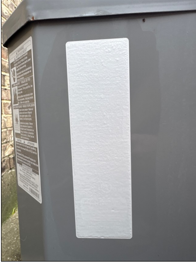
B. Item 4 Condensing Unit Data Label
