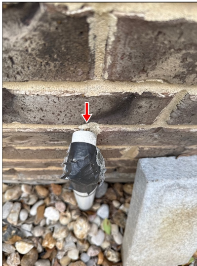
F. Item 7 Exterior wall penetrations need to be sealed at right side of garage
