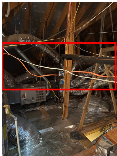
B. Item 2 Observed loose conductors in attic space
