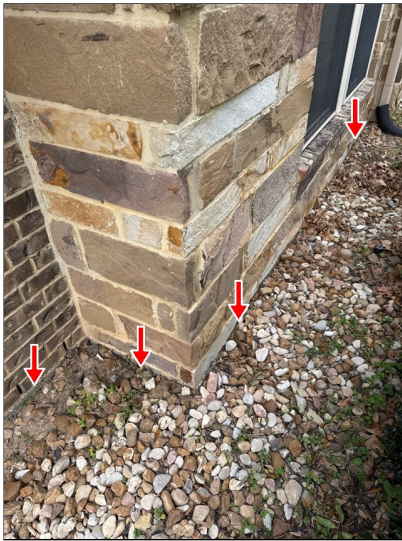
B. Item 3 High soil conditions observed at front of home, left of entry.
