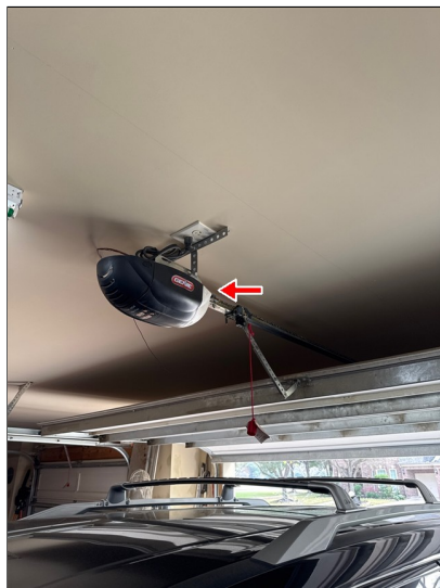
H. Item 1 The auto reverse on obstruction feature does not function normally at 2-car door
