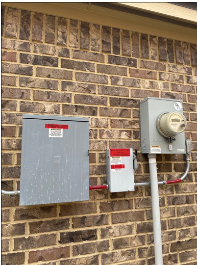
A. Item 6 The solar sub-panel box is located at the exterior right side of garage
