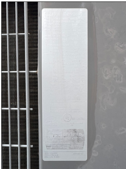
B. Item 1 Condensing Unit Data Label
