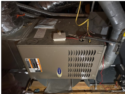
A. Item 1 The heating unit appeared to operate normally using the standard controls at primary system
