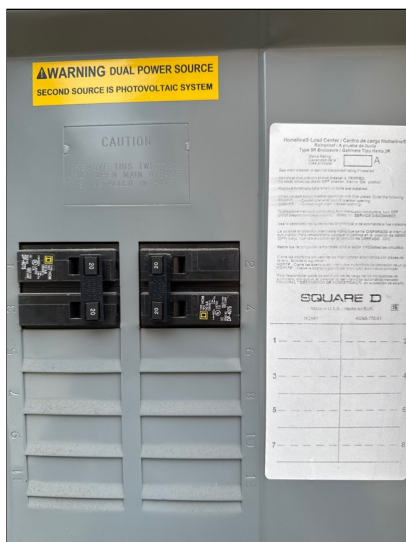
A. Item 4 No labels are present at solar sub-panel
