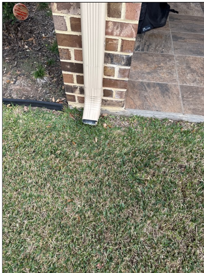
B. Item 1 Splash block or downspout extensions are absent at left rear corner of patio
