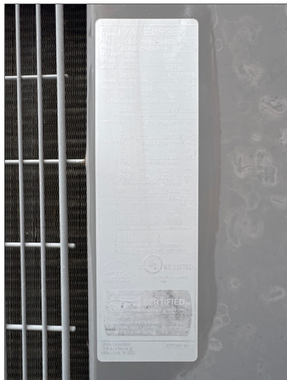
B. Item 1 Condensing Unit Data Label
