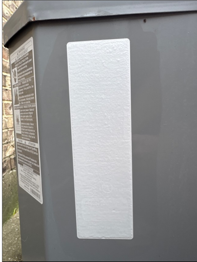
B. Item 4 Condensing Unit Data Label
