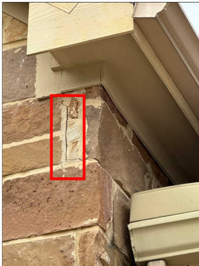
F. Item 8 Observed cracks in stone veneer at right side of entry
