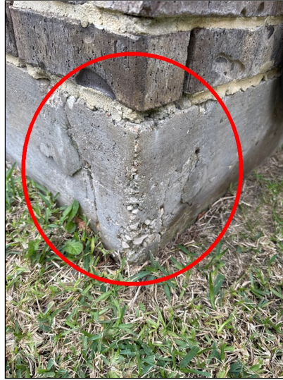
A. Item 3 Common corner crack observed at right rear corner of home
