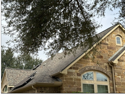
C. Item 7 This roof covering is probably around 5-7 years old and shows signs of wear consistent with its age, except as otherwise noted
