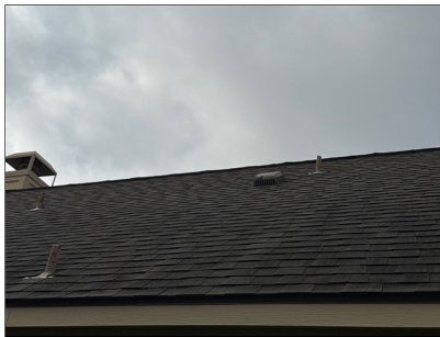
C. Item 12 This roof covering is probably around 5-7 years old and shows signs of wear consistent with its age, except as otherwise noted
