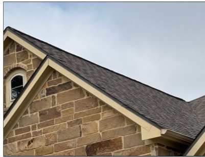
C. Item 4 This roof covering is probably around 5-7 years old and shows signs of wear consistent with its age, except as otherwise noted
