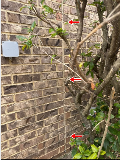
F. Item 5 The brick veneer expansion joint sealant has deteriorated at right side of garage
