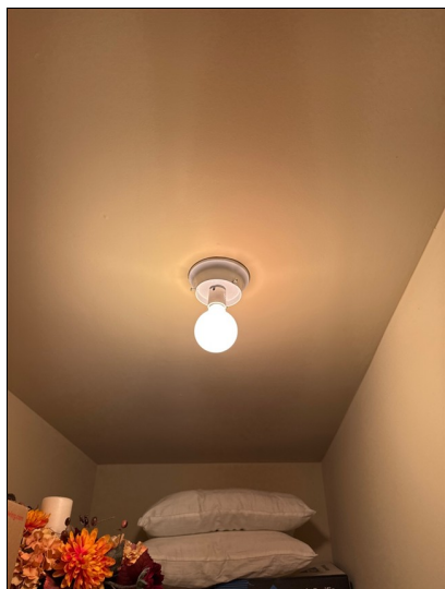
B. Item 1 Light fixture is missing globe/cover at front left bedroom closet
