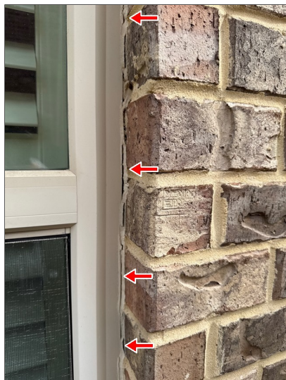
I. Item 1 The perimeter sealant has deteriorated at numerous windows throughout
