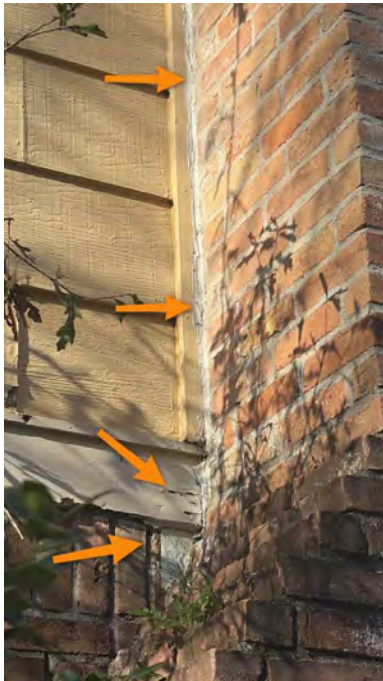
Right Side- mortar, damage, caulk
