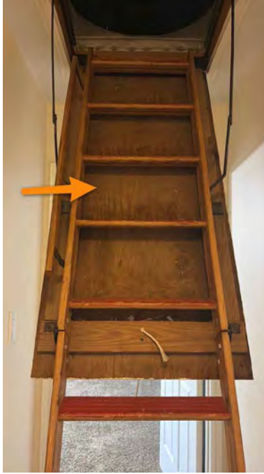
Main attic- missing insulation
