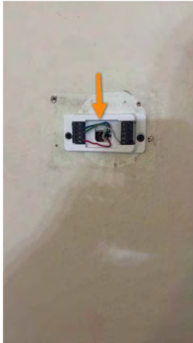
Thermostat uninstalled- unable to operate system
