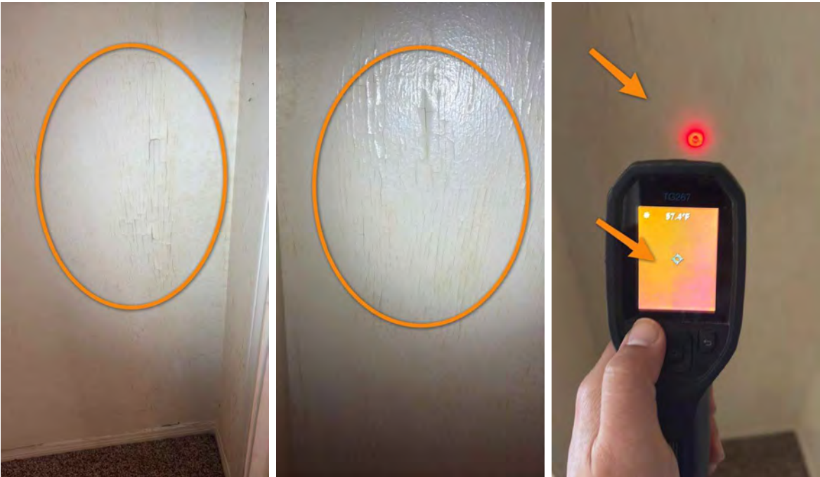
Coat closet 2- peeling paint indicates possible imposture penetration
