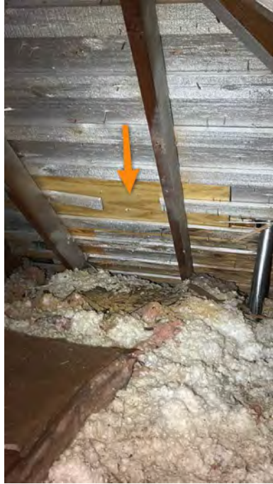
Bedroom 3 scuttle door- damaged
