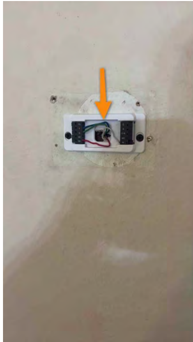
No thermostat, unable to operate system
