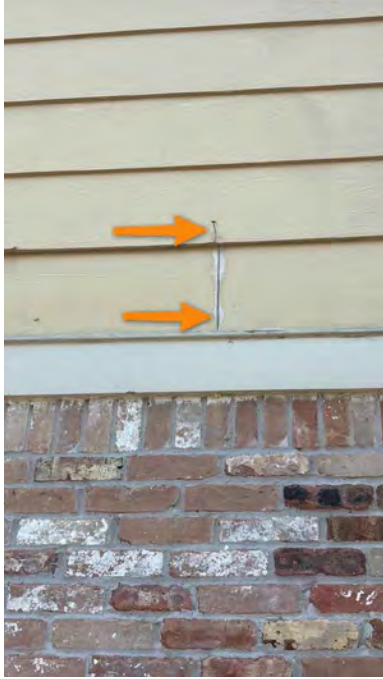
Left Side- damage and sealant
