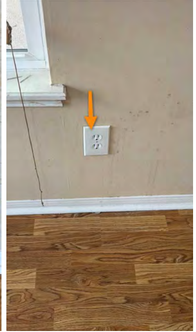
Kitchen Dining Room- loose
