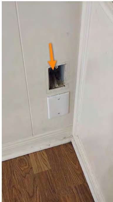
Living Room- missing
