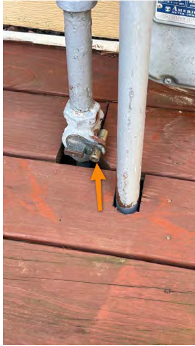
Gas off and locked
