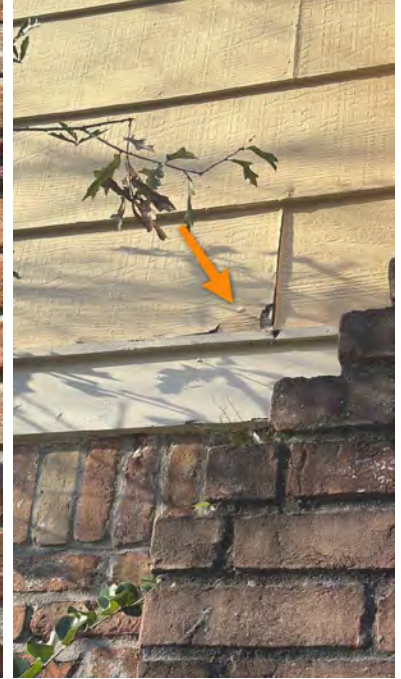
Right Side- damage
