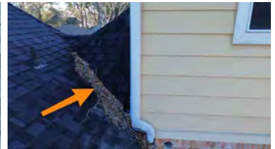
Left Side- debris
