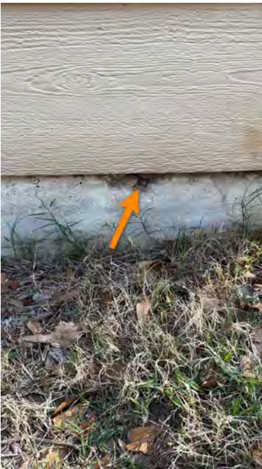
Left Side- chipped
