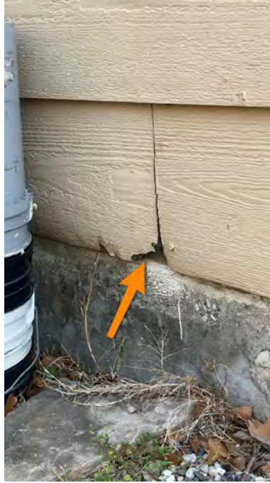
Left Side- deterioration
