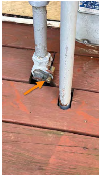
Gas off and locked at meter
