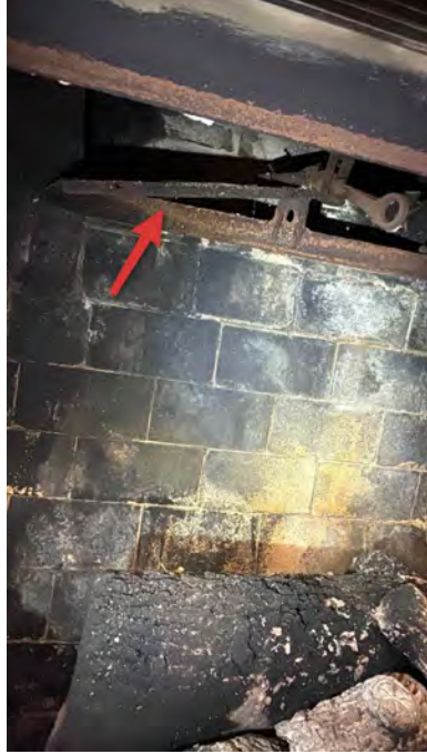
Rusted and not fastened to control mechanism
