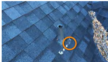
Left Side- exposed fastener
