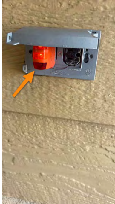
All exterior outlets
