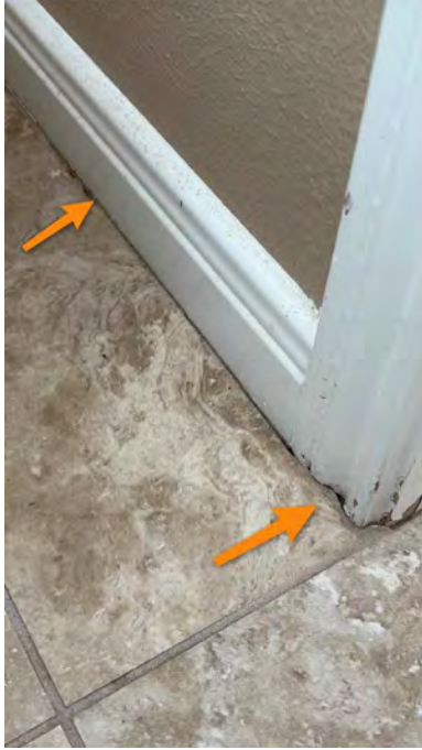
By Primary toilet
