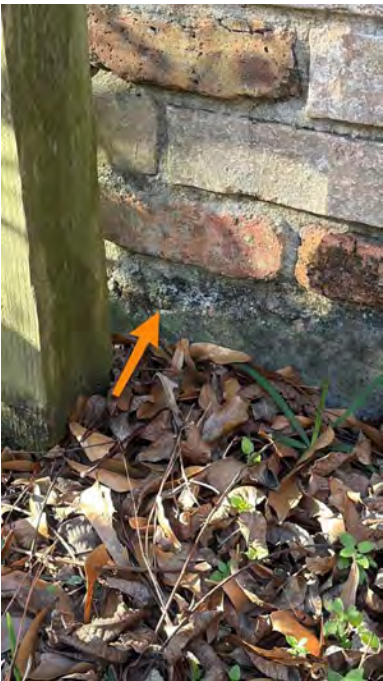
Right Side- chipped
