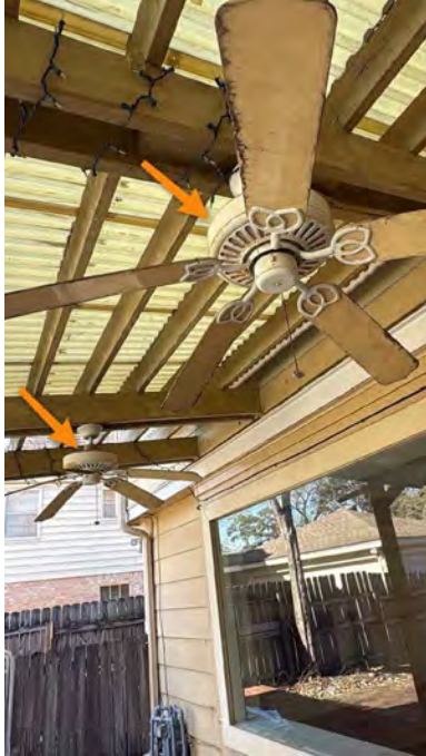
Back pario- rusted and blades warped
