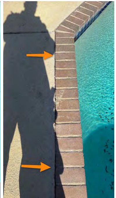
Missing around coping
