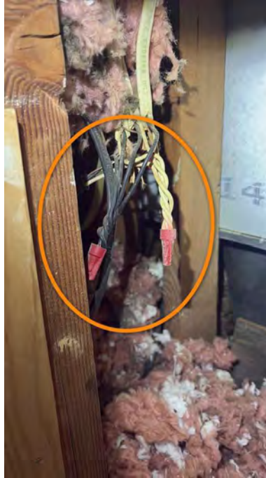
2nd floor plumbing access panel
