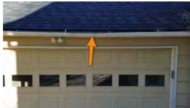
Above garage- damaged
