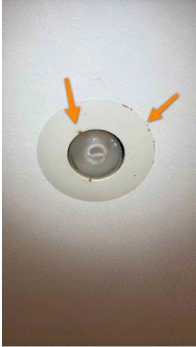
Primary bedroom- rusted
