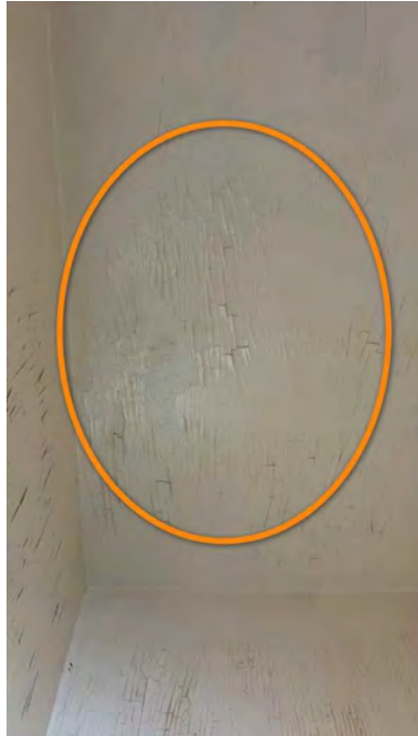
Cost closet 2- bubbling paint indicates moisture penetration
