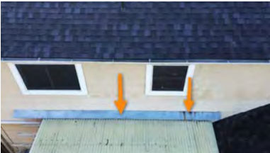
Rear- unpainted and rusted
