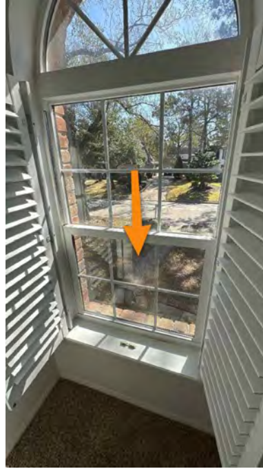
Bedroom 4 closet- does not stay up
