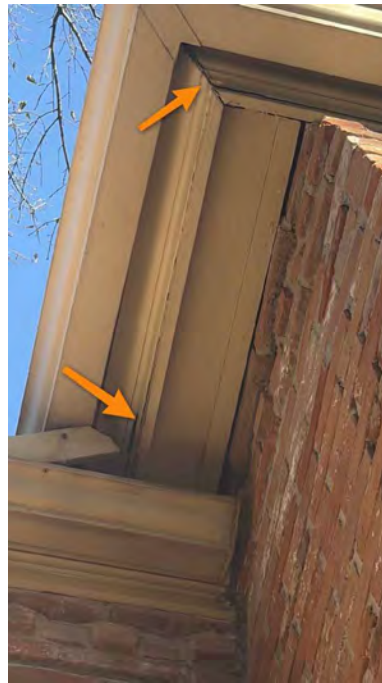
Front- sealant and damage
