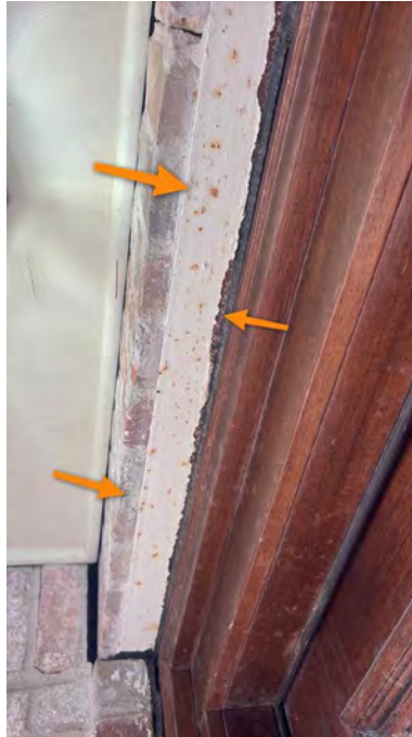
Above front door- rust
