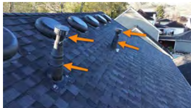
Rear- insufficient height and missing storm collar
