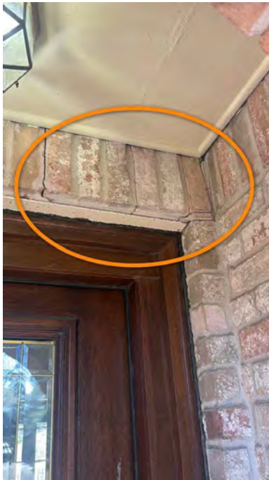
Above front door-mortar cracks
