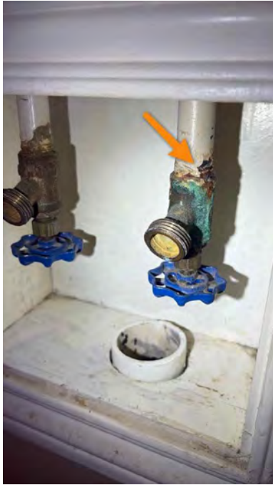
Washing machine supply lines
