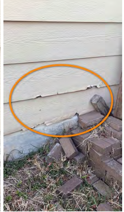
Left Side- deterioration
