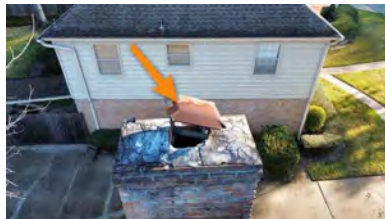
Rusted and not fully seated property
