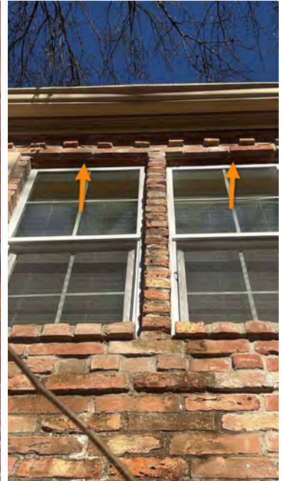
Front Left- rust
