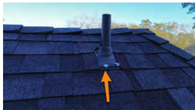
Above garage- lifted shingle
