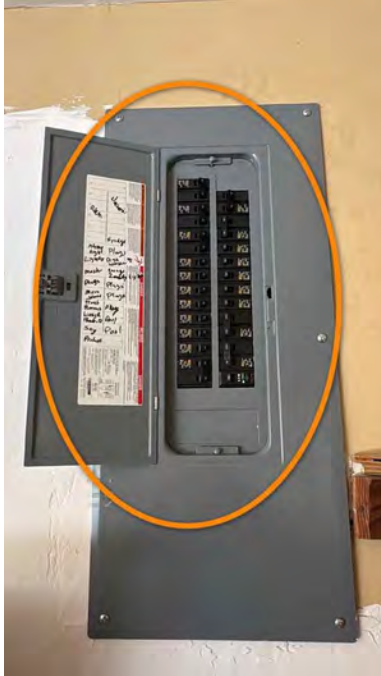
No disconnect installed or observed
