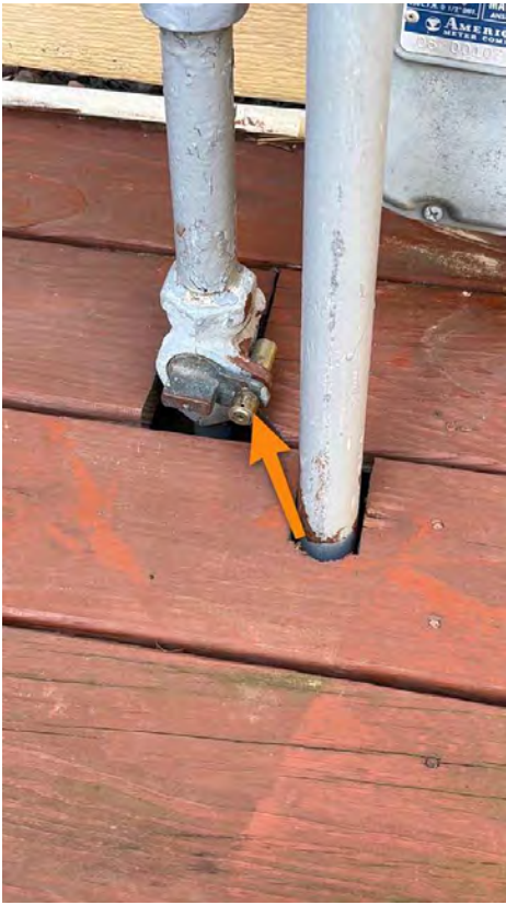
Gas off and locked at meter
