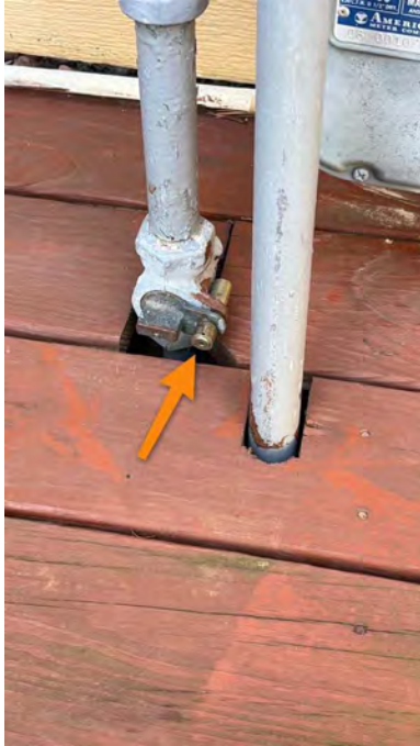
Gas off and locked at meter
