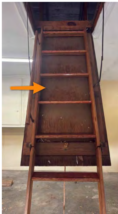
Garage attic-missing insulation
