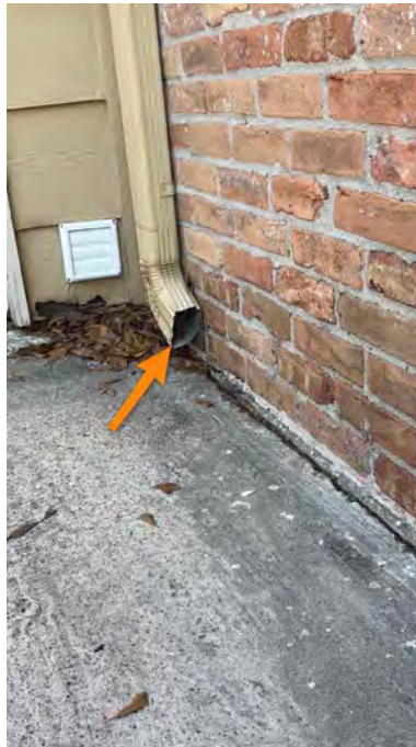
Left Side- elbow should not discharge along foundation
