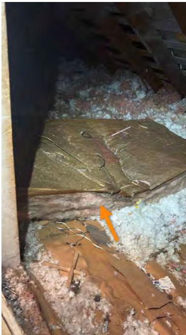
Bedroom 3 scuttle door- improper install
