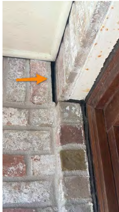
Above front door- missing mortar/opening
