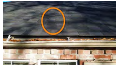
Front left- lifted shingles
