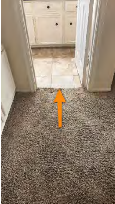
2md floor hallway- sloped into bathroom
