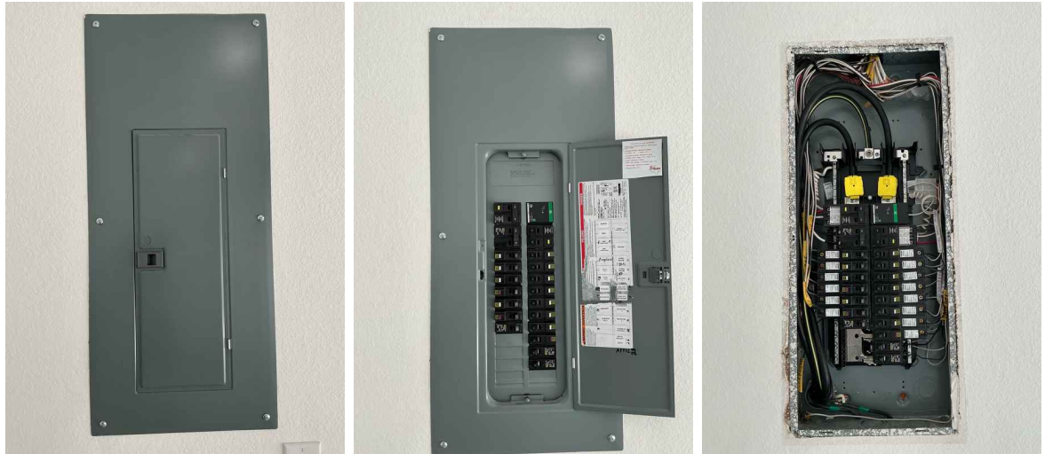
Photo of distribution panel: Garage
