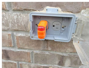
Exterior Receptacles - not trip
