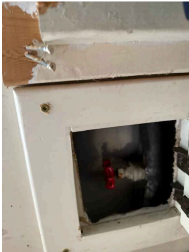
Photo of Type of Supply Piping Material: PVC, CPVC
