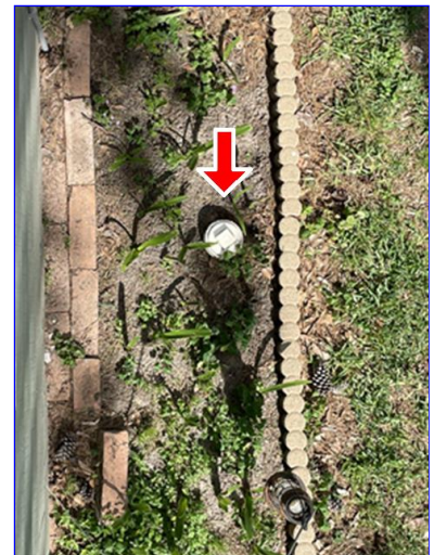
B. Item 4(Picture) PVC clean out
