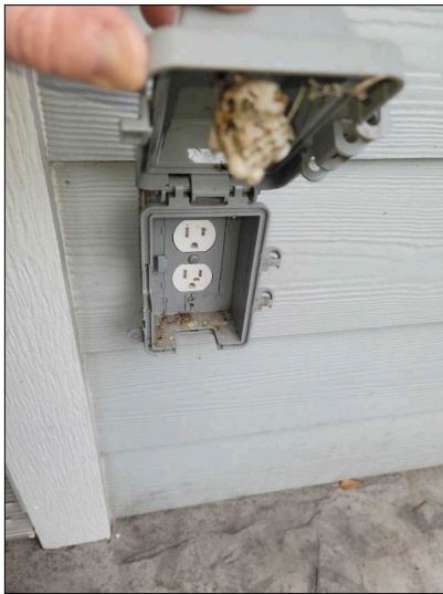
No GFCI protection at outdoor outlet.. rear
