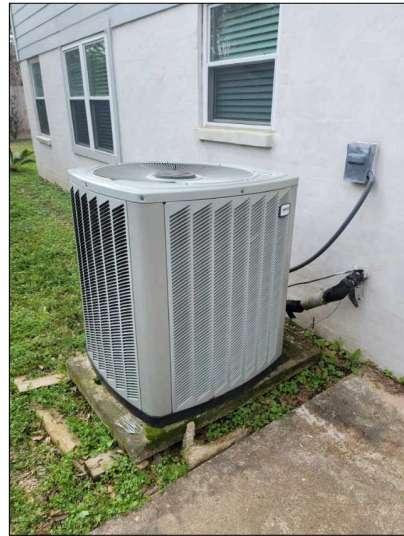
Upstairs (left side) AC compressor, label indicates R22 refrigerant, 4 ton unit, manufactured July 2006. Rated for 40 amp maximum, may be fed by 50 amp breaker.
