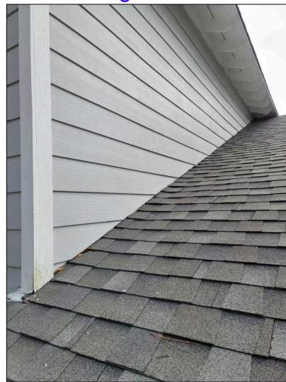
Wall lacks minimum 1" clearance from shingles..right side
