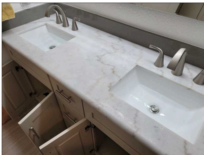
Slow draining sinks in several locations
