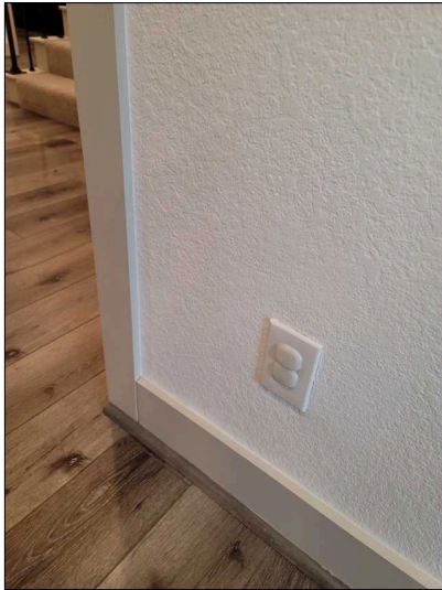
Loose outlet..breakfast area
