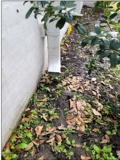
Missing splash block..front right
