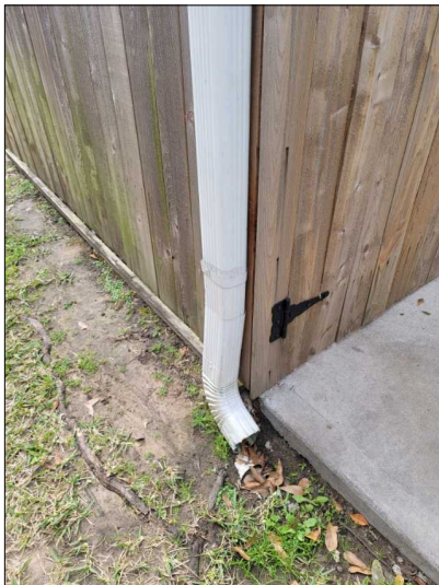
Missing splash block..front left
