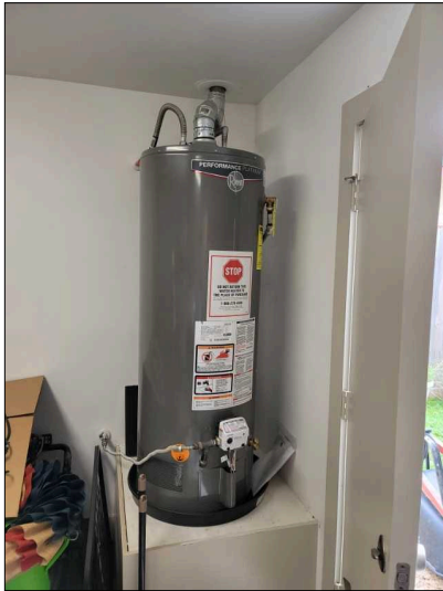
50 gallon gas water heater in garage, manufactured Nov 1019.
