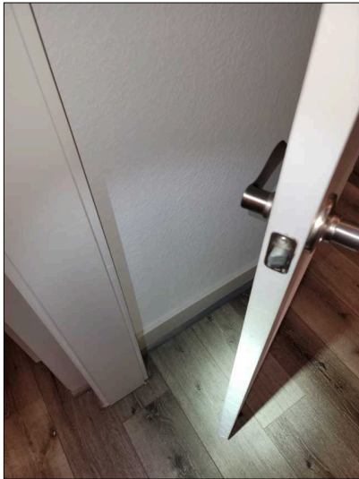
Missing door stop..laundry
