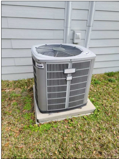
Downstairs (right side) AC compressor, R22 refrigerant, 3 ton unit, manufactured June 2009. Rated for 30 amp maximum, fed by 40 or 50 amp breaker.
