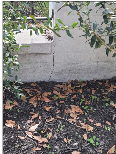
Brick crack at front patio wall.. front
