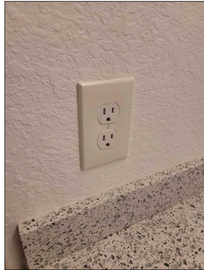
No GFCI protection at garage bathroom outlet
