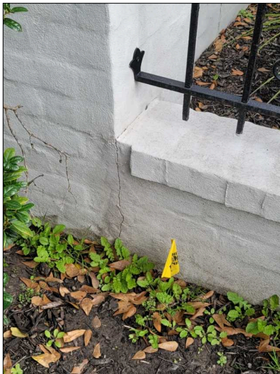
Brick crack at front patio wall.. right side
