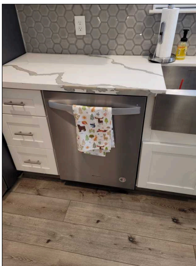
Dishwasher operational, lacks electrical disconnect
