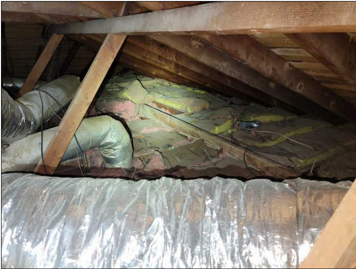
Missing, compressed insulation in several areas..upper attic
