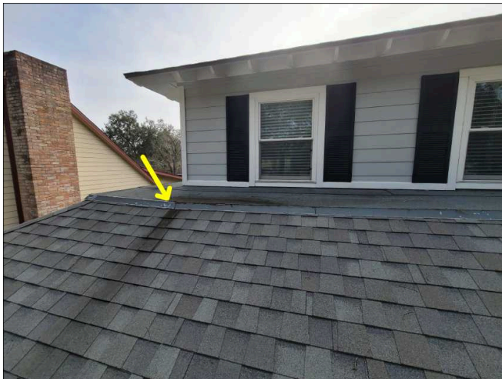
Sag evident above garage
