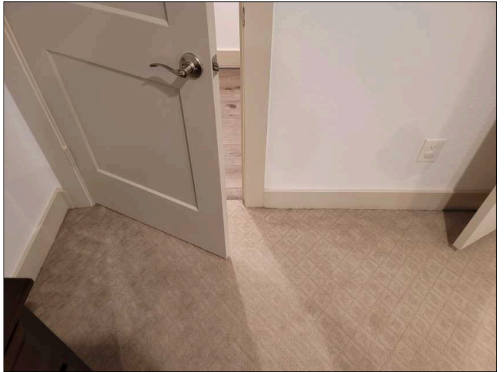
Missing door stops..primary bedroom
