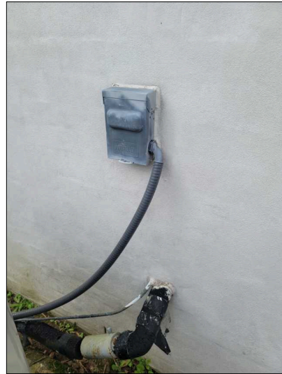
Disconnect behind unit..left side
