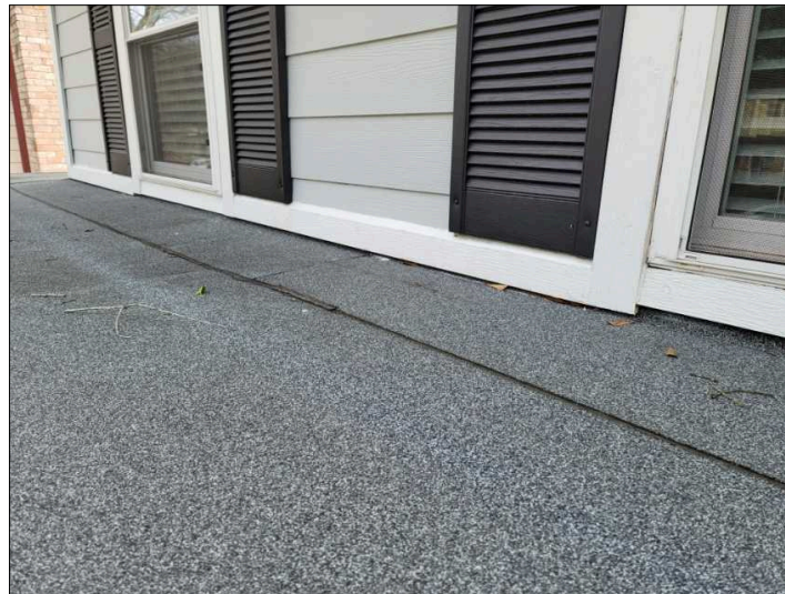
Wall lacks proper clearance from roofing material.. front
