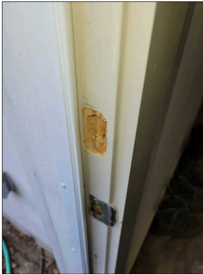
Missing deadbolt strike plate.. garage rear door
