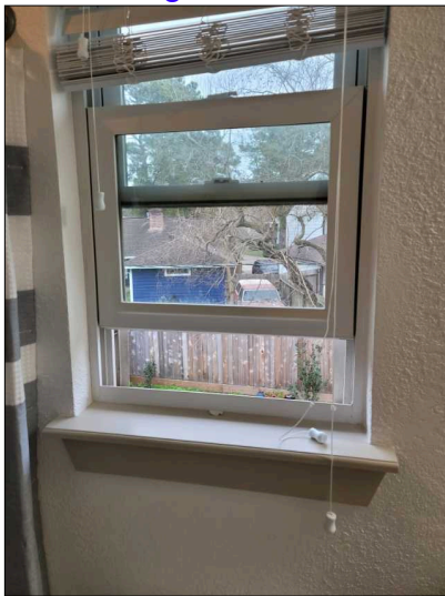
Missing screen..upstairs rear left bathroom
