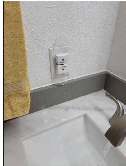
No GFCI protection at sink outlets.. left upstairs bathroom
