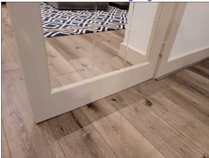
Dining/living room door rubs at floor
