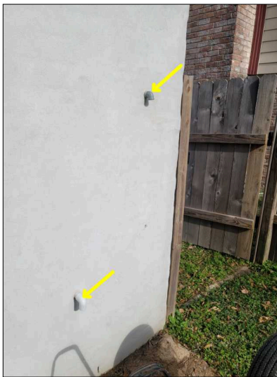
Water heater drain lines too high, should be within 6" of grade to avoid scalding.. rear of garage
