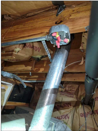
Junction box missing cover..lower attic
