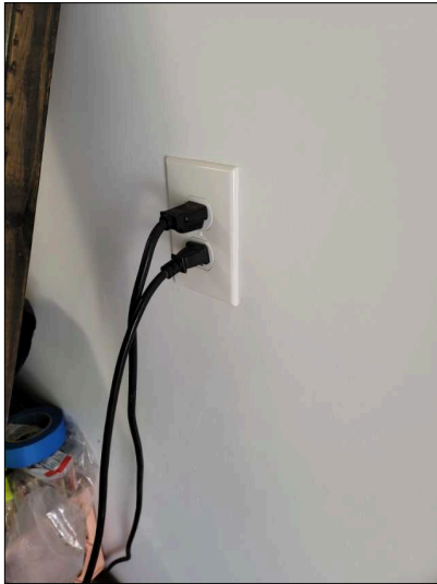
No GFCI protection at garage outlets
