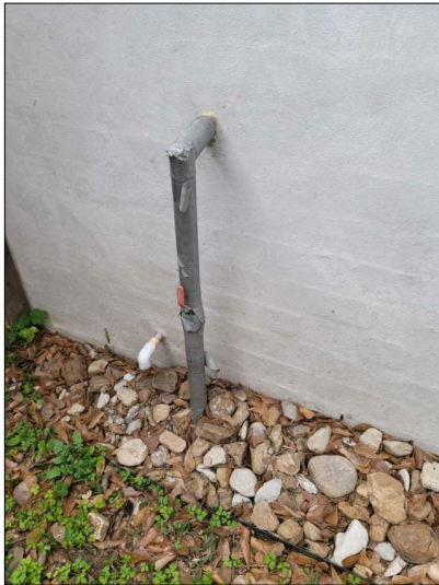
Water shutoff..left side
