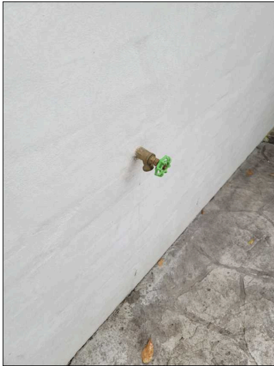
Hose bib lacks backflow preventer..front
