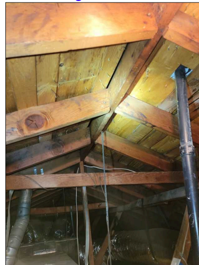
Ridge beam too small, lack of adequate ventilation..upper attic
