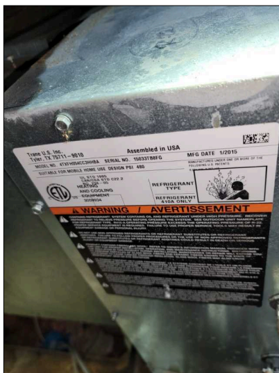
Upstairs (upper attic) AC evaporator coil, label indicates R410A refrigerant, manufactured Jan 2015, approx 18F temperature differential
