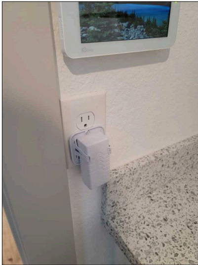
No GFCI protection at laundry sink
