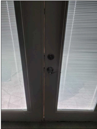
Double doors not sealing..primary bedroom
