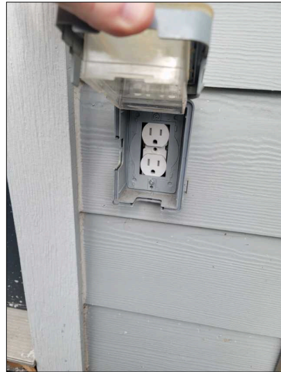
No GFCI protection..back door
