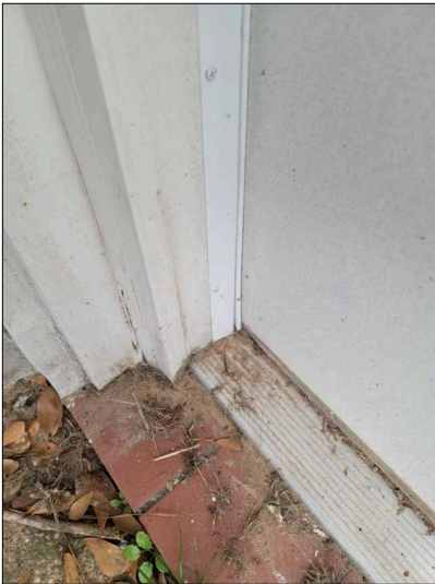
Rotted wood trim..rear garage door
