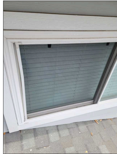
Damaged screen frame.. right side
