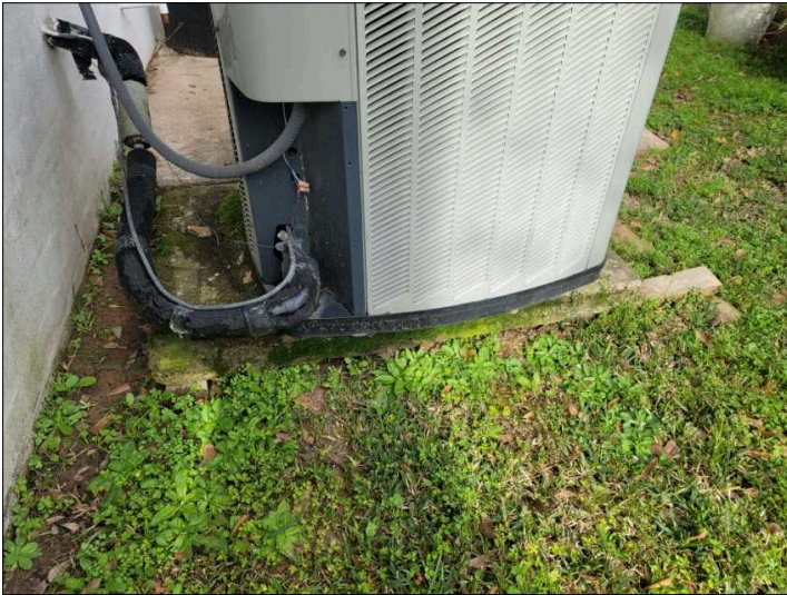
Wood to ground contact under AC unit near left side wall
