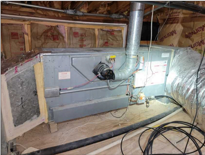
Downstairs gas furnace (lower attic), old unit, rusted heat exchanger needs to be evaluated by HVAC contractor
