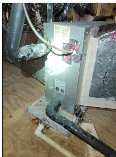
Downstairs AC evaporator coil (lower attic), manufactured April 2004, 8F temperature differential. Lacks secondary drain line
