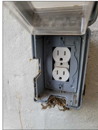
No GFCI protection..front door
