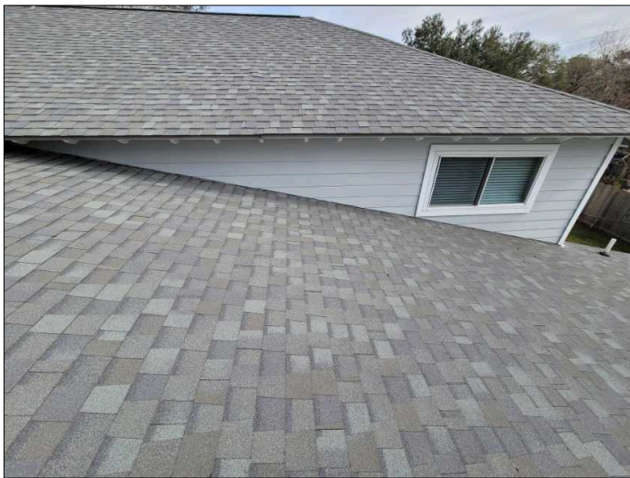
Wall lacks minimum 1" clearance from shingles..right side
