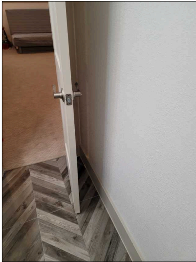
Missing door stop..upstairs rear left bathroom
