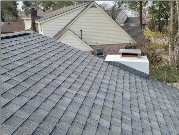
Chimney height inadequate. Should be minimum 3' above shingles and 2' above any structure within 10'
