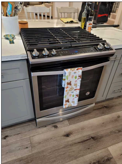
Gas oven/range, shutoff appears to be behind unit. Inaccessible in an emergency.
