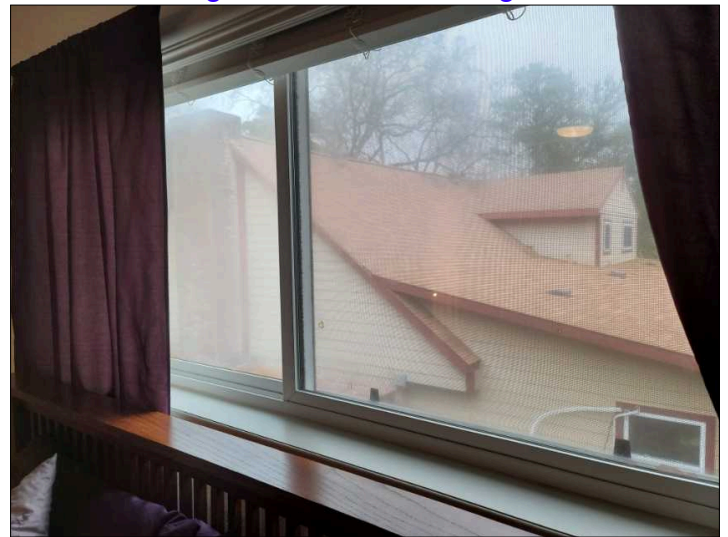
Fogged windows..rear left upstairs bedroom
