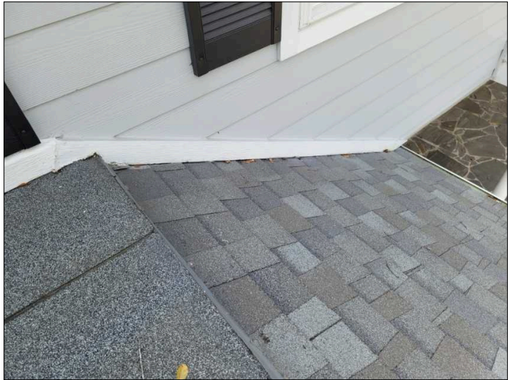
Wall lacks minimum 1" clearance from shingles..front
