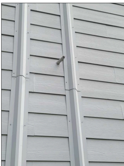
Info..AC secondary drain line..right side
