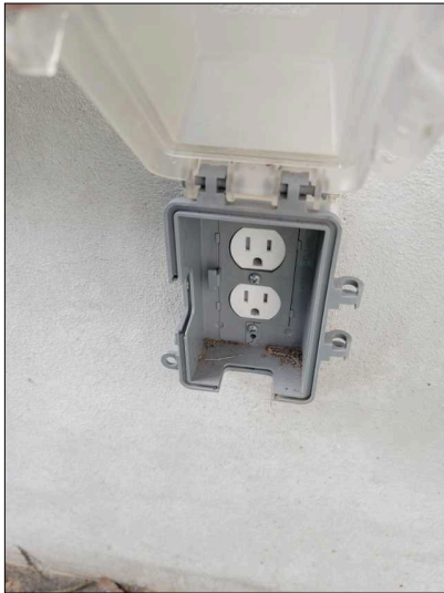
No GFCI protection at outdoor outlet..rear garage door
