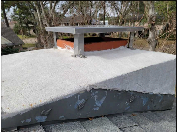
Lacks spark arrestor
