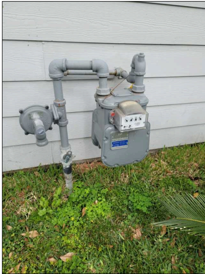
Gas meter and shutoff.. rear
