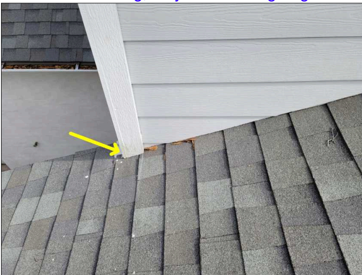
Missing kickout flashing.. right
