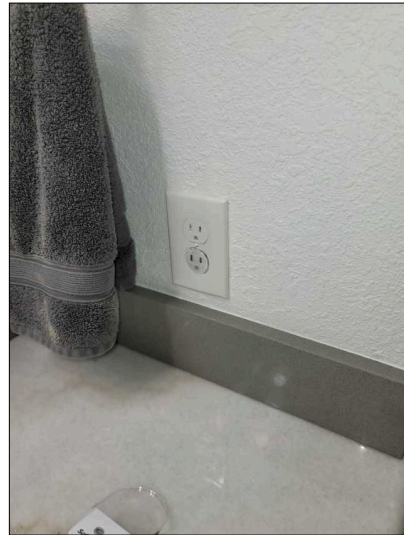
No GFCI protection upstairs rear left bathroom
