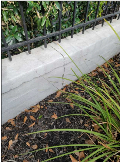
Brick crack at front patio wall.. front
