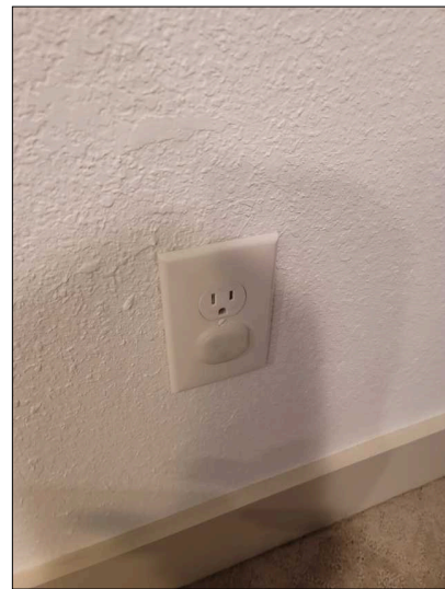
Loose outlet..primary bedroom
