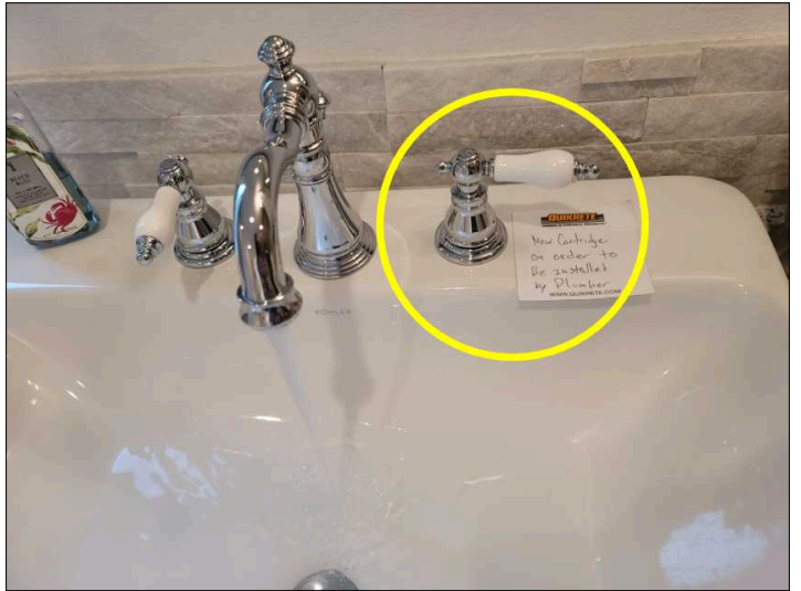
Left side sink, no cold water supply..primary bathroom
