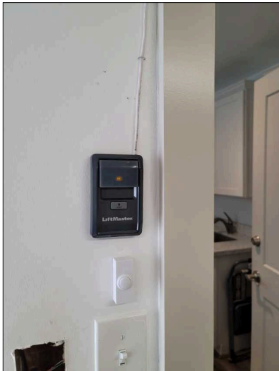
Missing safety instructions
