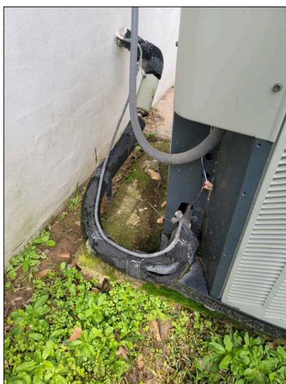
Missing insulation on AC cold line..left side
