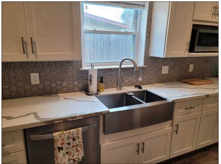
No GFCI protection at kitchen sink outlets, loose right outlet
