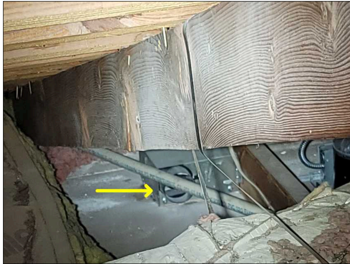
Bathroom exhaust venting into upper attic
