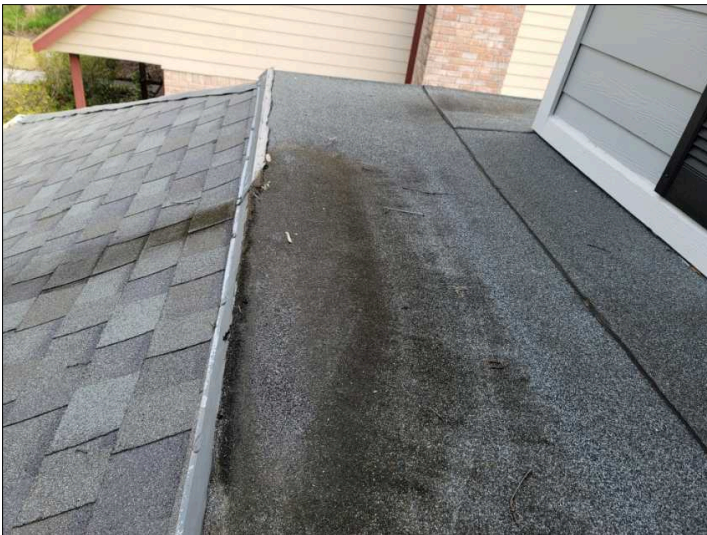
Low sloped section appears to be holding water, lifted flashing, may leak.. over garage
