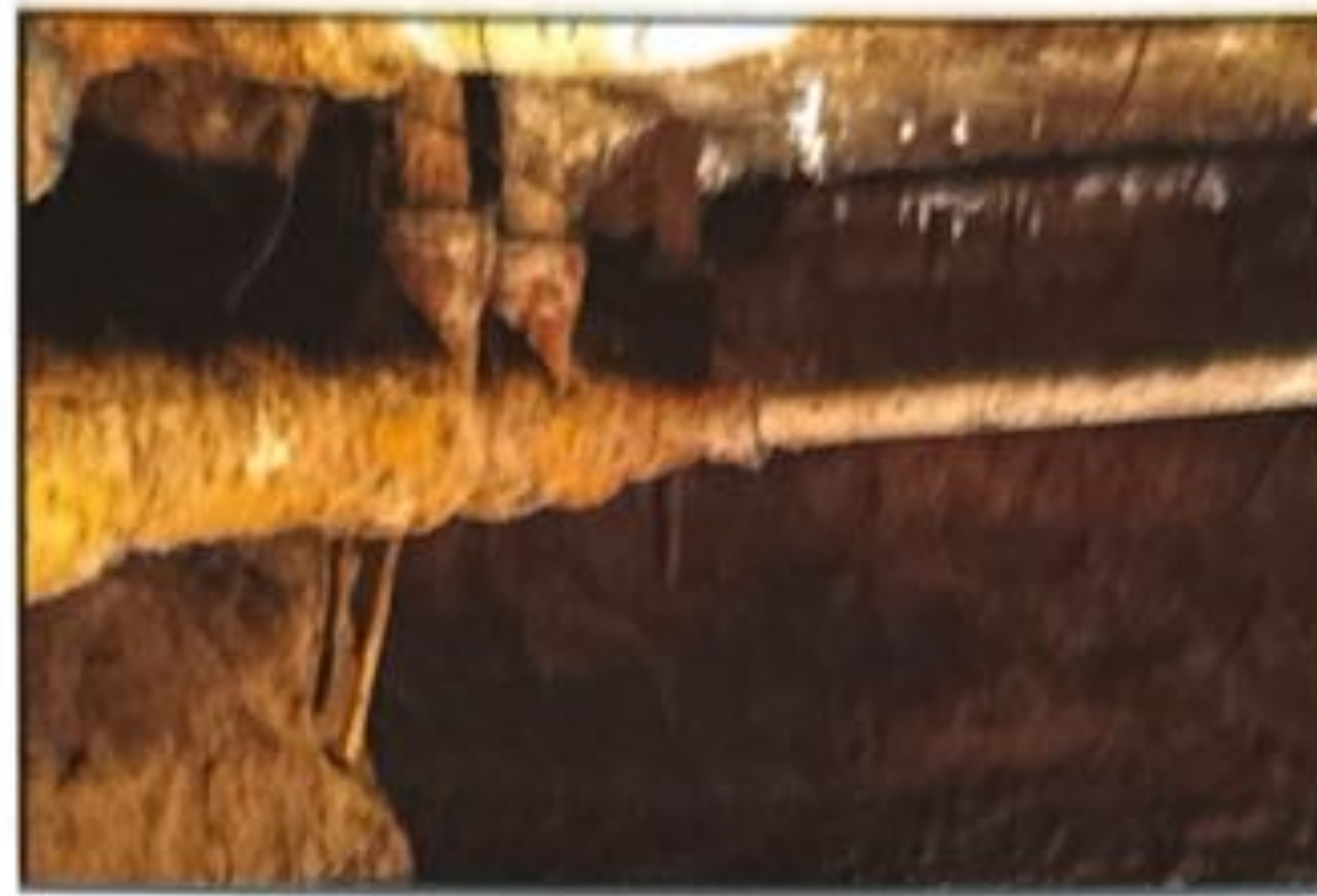
CAST IRON/ABS PIPES SEWER LINE FAILURE
