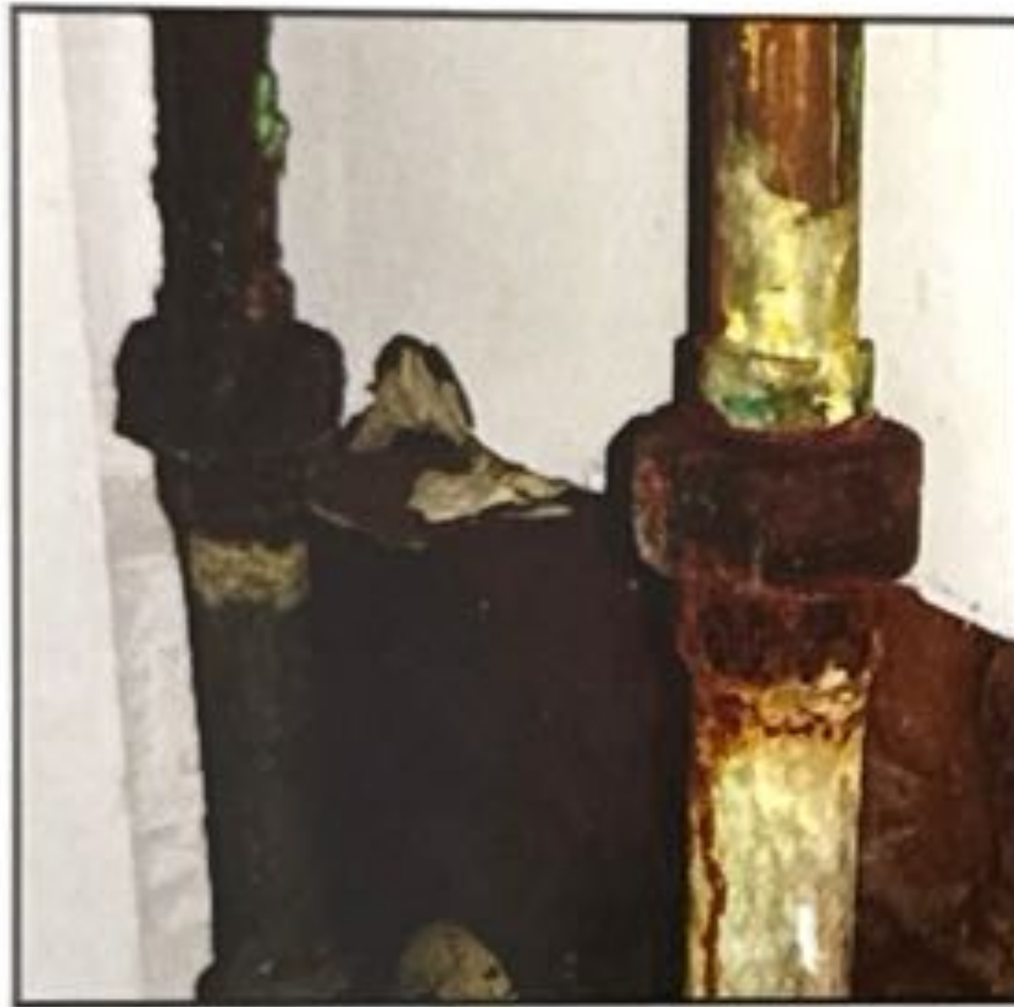
LOW PRESSURE DAMAGING LEAKS
