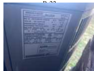
American Standard 4 ton built in 2019, min/max breaker 25/40 amps, R-410A
