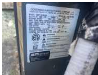
Goon 3 ton built in 2015, min/max breaker 20/30 amps, R-410A
