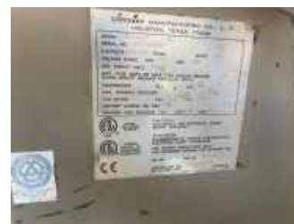
Goodman 1.5 ton built in 2003, min/max breaker 10/20 amps, R-22
