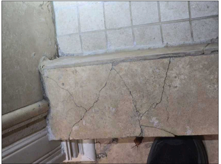
Floor tile of shower curb is broken in several places.
