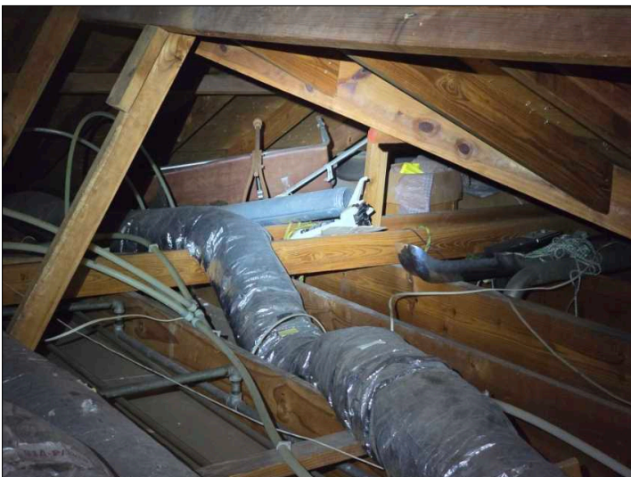
Heavy debris and belongings left in attic space noted.
