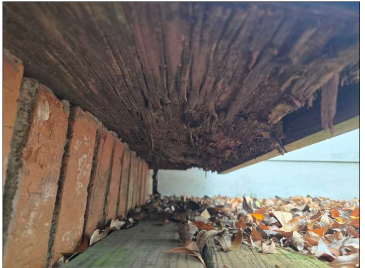
Wood rot / termites damages at wall alcove.
