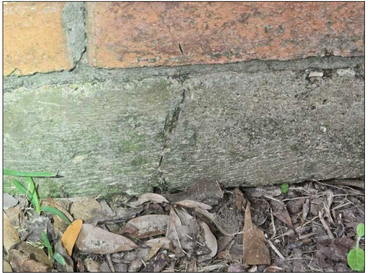
Exterior cracks in foundation noted. 2 found.
