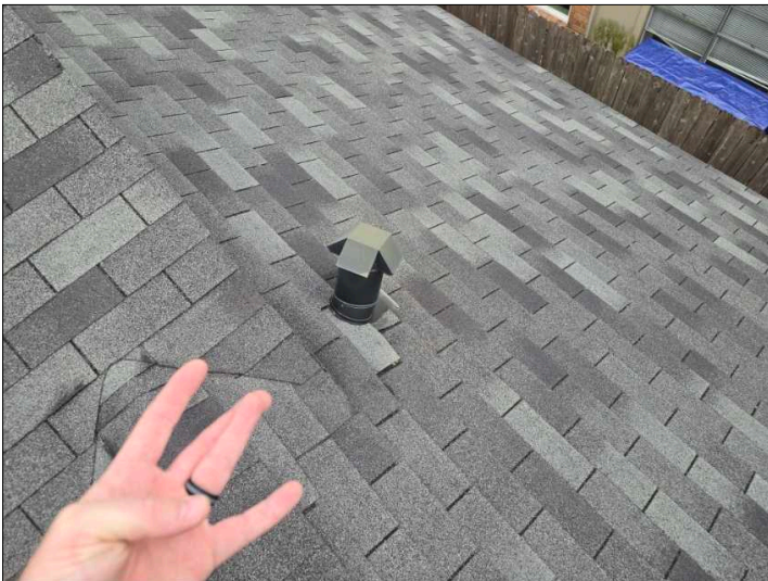
Incorrect furnace /water heater exhaust vent pipe. Should be a double wall type B vent and cap above roofline.
