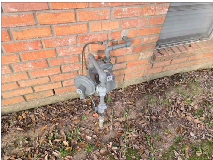
Gas Meter and Shutoff Location.
