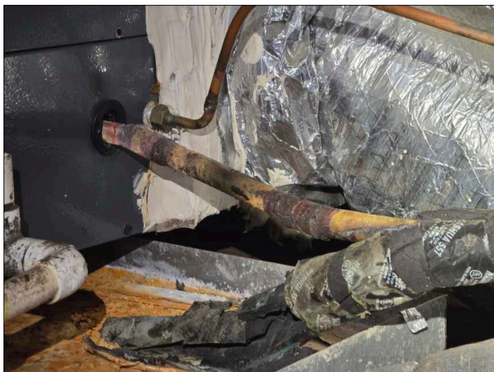
Coolant lines missing insulation in attic space. This will condensate and drip onto attic floor / ceiling.
