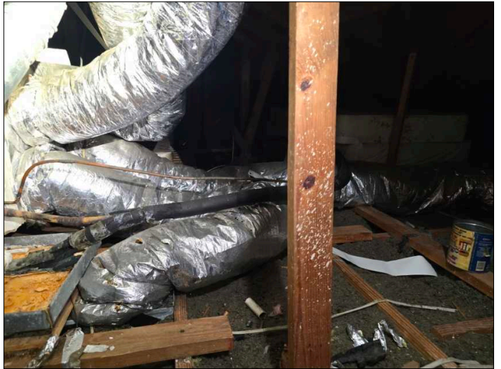
90 degree bend in flex lines present. This restricts air flow and balance of conditioned air in home.
