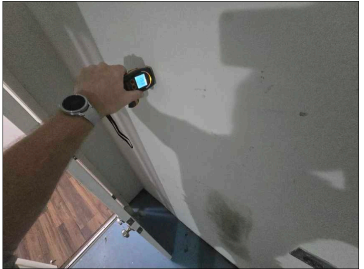
Moisture damages noted in wall of garage. Moisture detected.
