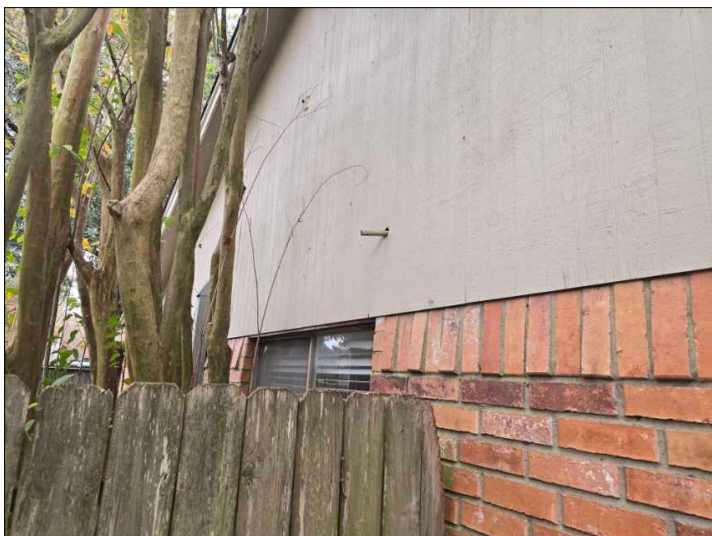
Secondary Drain line discharge location is over window. If water is seen coming from here, the primary may be stopped up. Contact HVAC service immediately to prevent possible damage.
