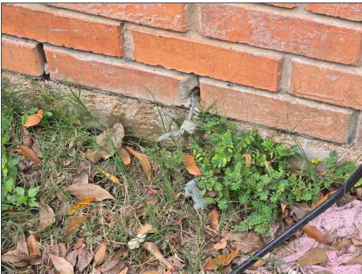
Ground rod is disconnected from the grounding conductor. This should be repaired.
