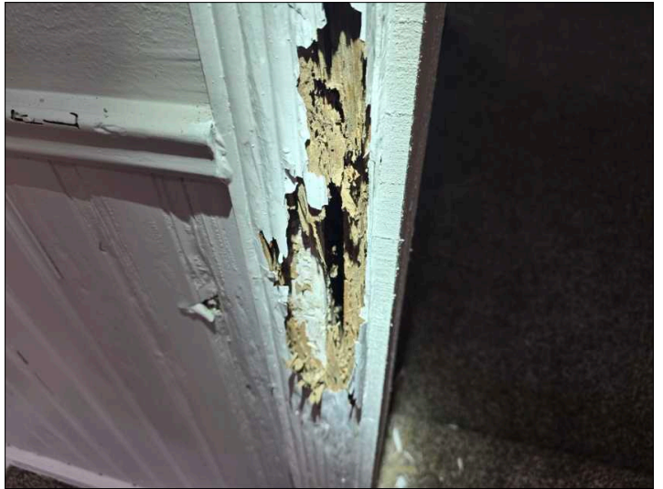
Extensive damage to rear of house. Deck, back room, and walls are all likely going to need to be opened to check for damages and repair.
