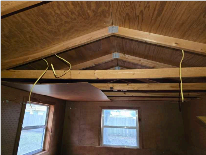
Unfinished electric to shop. No power to panel.
