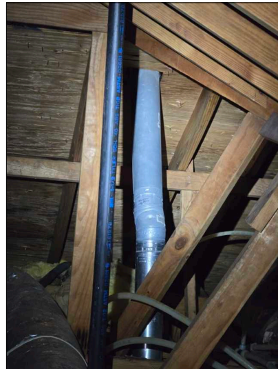
Flues are missing metal strapping.
