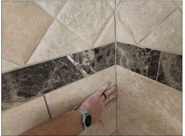
Cracks in tile grout at tub area. Suggest sealing these areas
