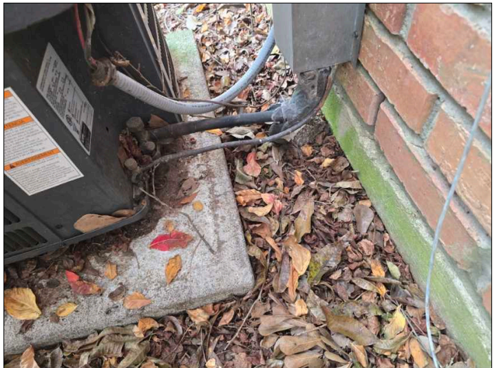
Refrigerant lines are missing insulation at the A/C unit
