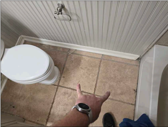
Crack in floor of 2nd bath. Appears to be foundation related.
