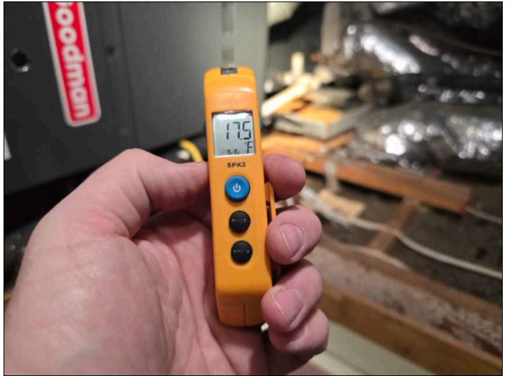
17f delta T across coil is acceptable.
