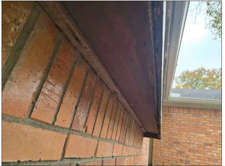
Wood rot in several places.
