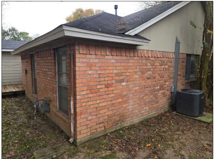
Recommend a Gutter system to aid in drainage away from house.
