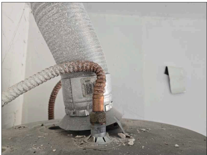
Damaged water line at water heater.
