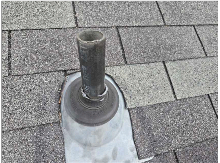
Vent boots are dry and broken. Leaks will occur. Repairs needed.
