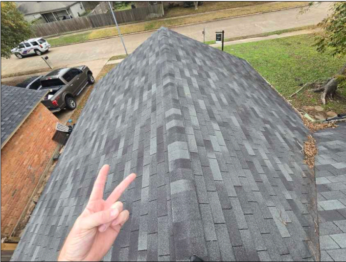
Ventilation is inadequate over garage.
