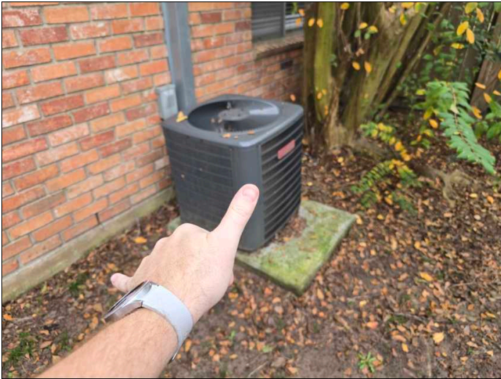
Exterior condensing unit should be resting level. Not currently level
