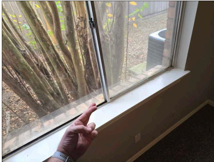
Window did not open in several locations.
