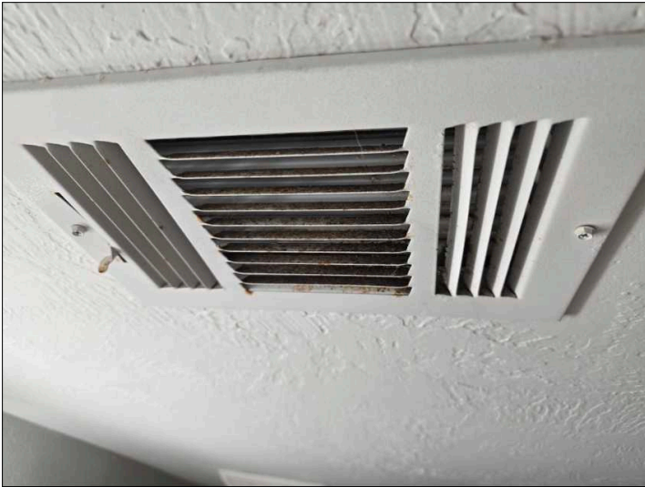
Rusted register noted in bathroom.
