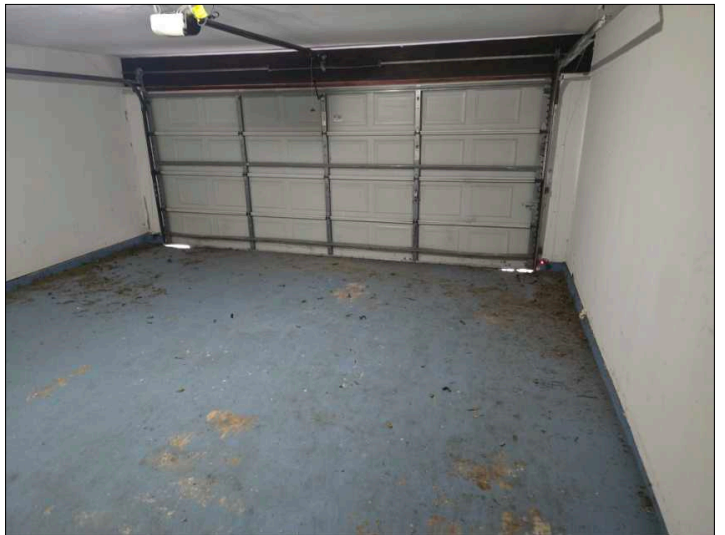
Garage door seal is damaged.
