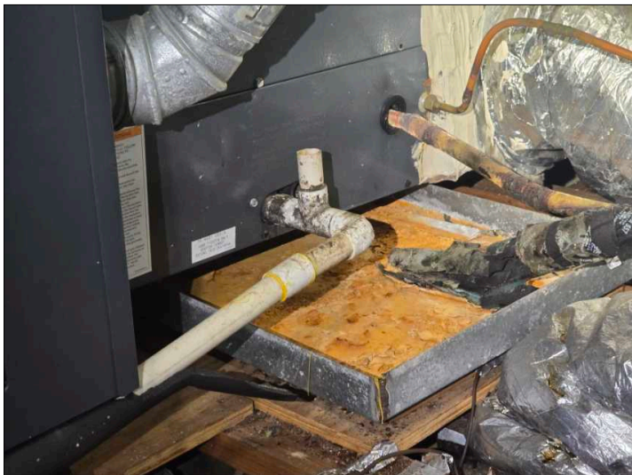
No secondary drain installed. This should drain into a catch pan if the primary is clogged.
