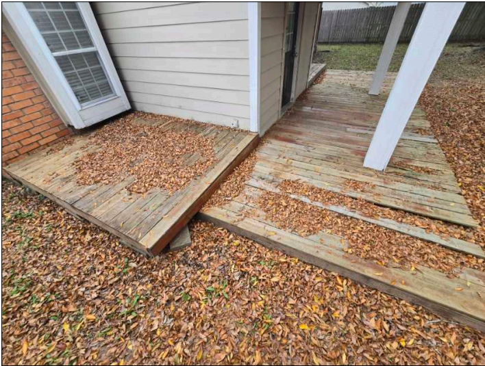
Deck in direct contact with earth. This is a possible location for wood destroying insects to enter.
