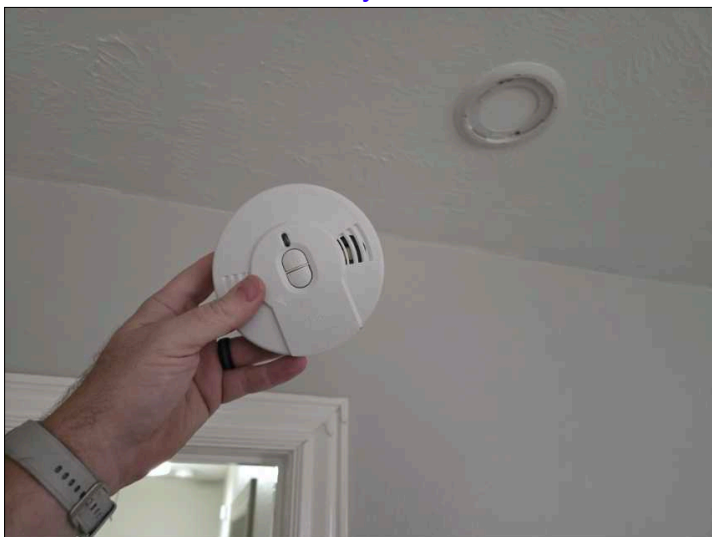
Smoke detectors not tied to other and missing CO detector.
