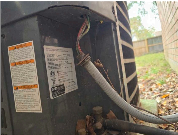
Conduit disconnected at AC unit.
