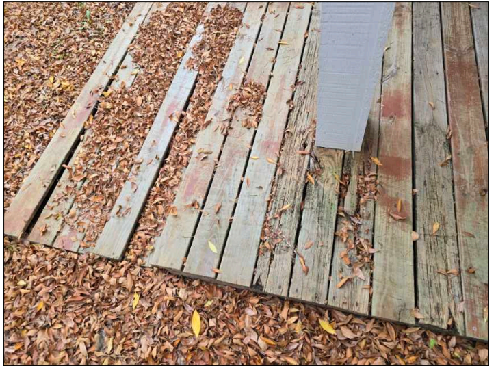
Termite damages, wood rot and trip hazards.
