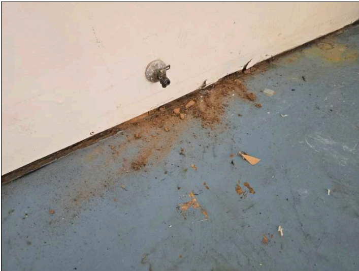
Ant and wall damages in garage.
