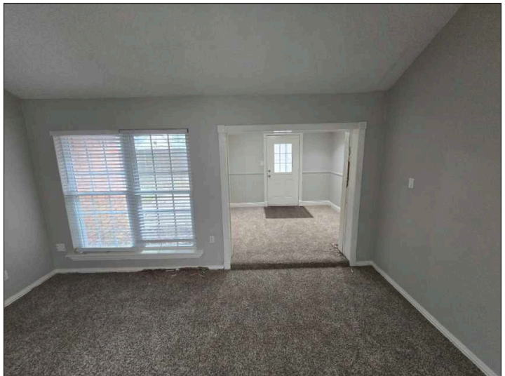
Active termite damages appear to stretch from kitchen to master bedroom. Heavy repairs and demo will be needed.
