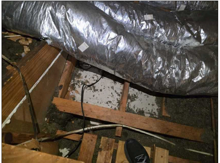
Missing insulation in several places.
