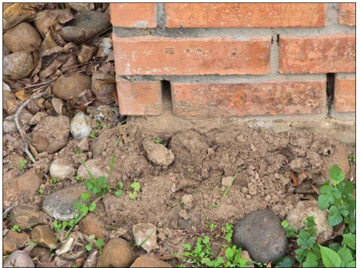
Ants entering walls.
