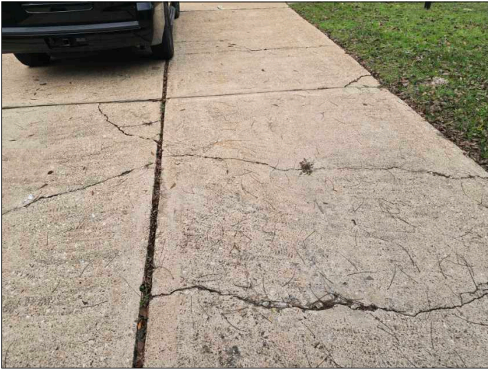
Driveway / sidewalk is cracked / lifted and has some tripping hazards.
