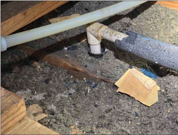
Main drain is tied to an open vent line in the attic. This is a risk of water overflow and damages. Plumber should seal connections.
