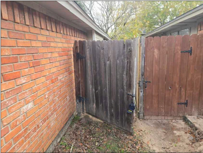
Gates are damaged and not fully functional.
