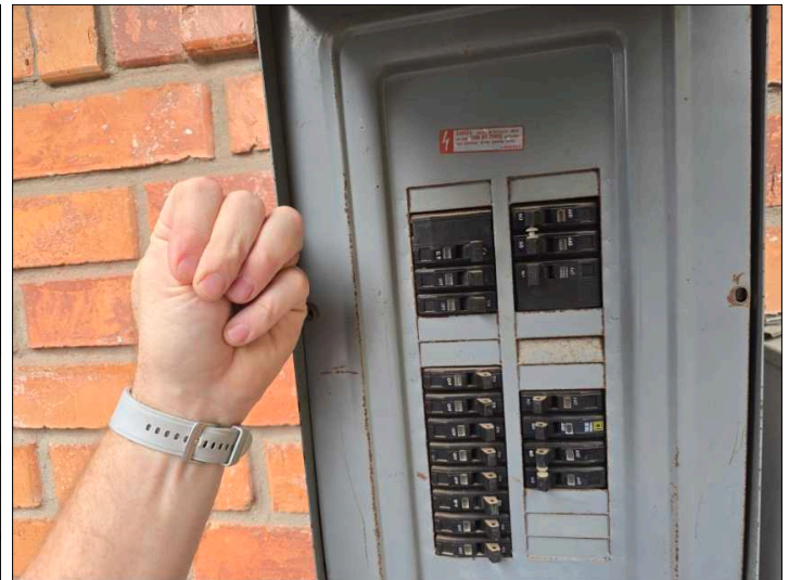
No main disconnect. Falls under old 4 throws of the hand rule.
