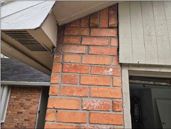
Recommend exterior siding weather proofing
