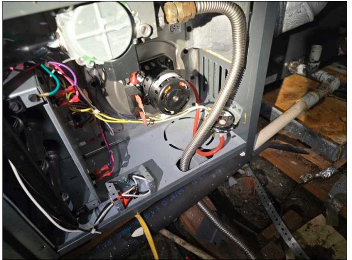
Flex gas line entering furnace cabinet is a fire hazard and should be corrected.
