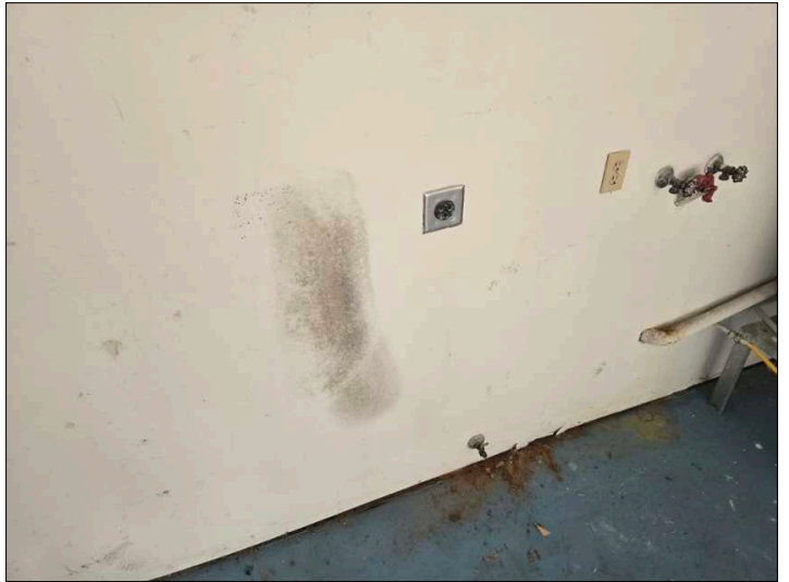
Mold damages along wall of garage.
