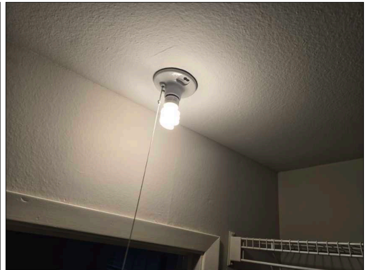
Open bulb light fixtures in closets are not allowed. Should be covered to reduce risk of fire.
