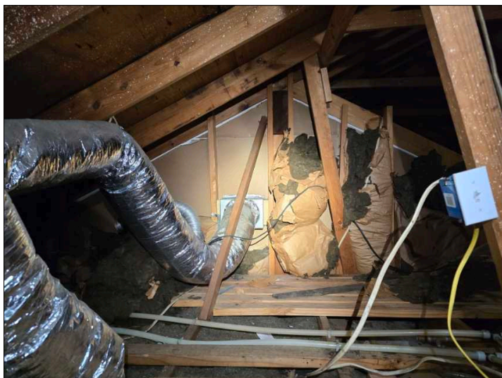
Missing insulation in several places.
