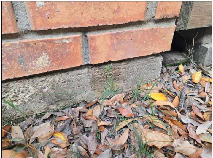
Active leak at drian in kitchen. Water flows freely from wall when sink/ dishwasher are running. Exact reason is unknown. Possible broken / clogged pipe or under ground blockage. Repairs needed.
