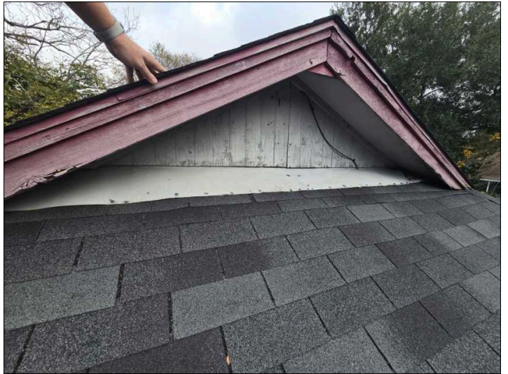
Multiple locations of deterioration around soffit and eave. Wood rot is subject to WDI
