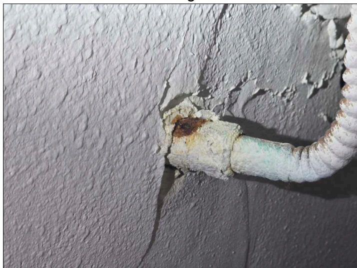
Home appears to have been repiped, but some rusted galvanized still present near water heater.
