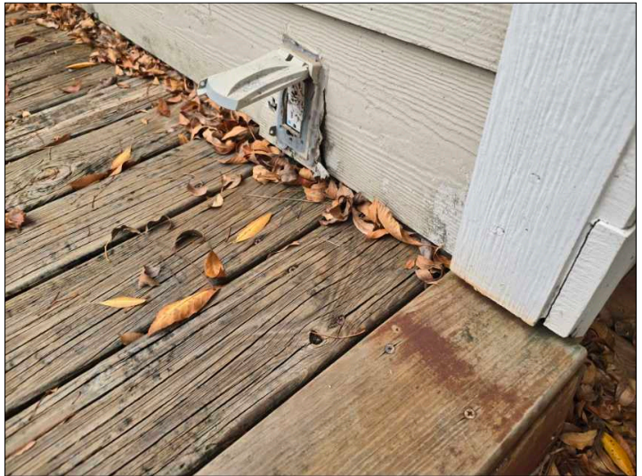
Loose receptacle found.
