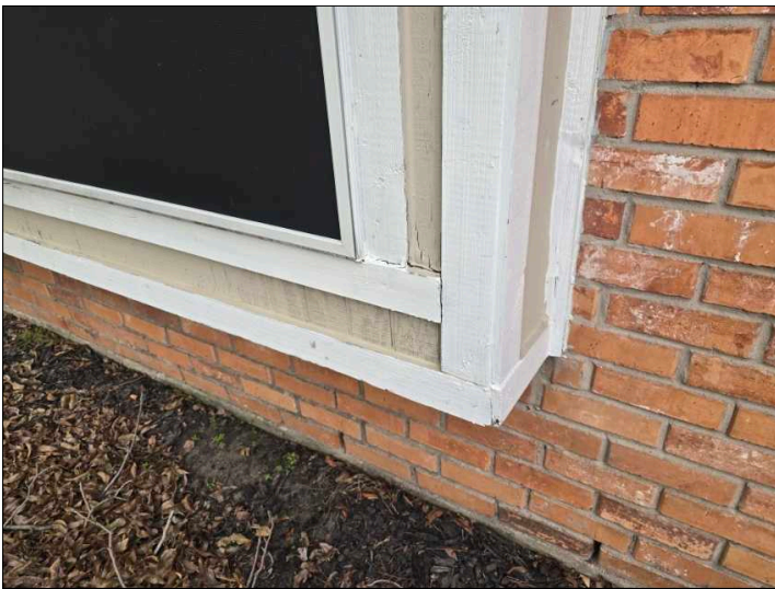
Wood rot in several places.
