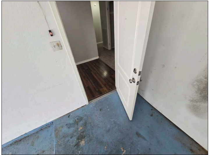
Garage door should have self-closing hinges that close door from wide open. Adjust hinge setting.
