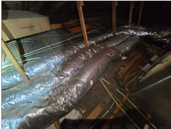
Flex ducting in contact with blown in insulation. This can cause mold growth. Flex ducting should be fully suspended.
