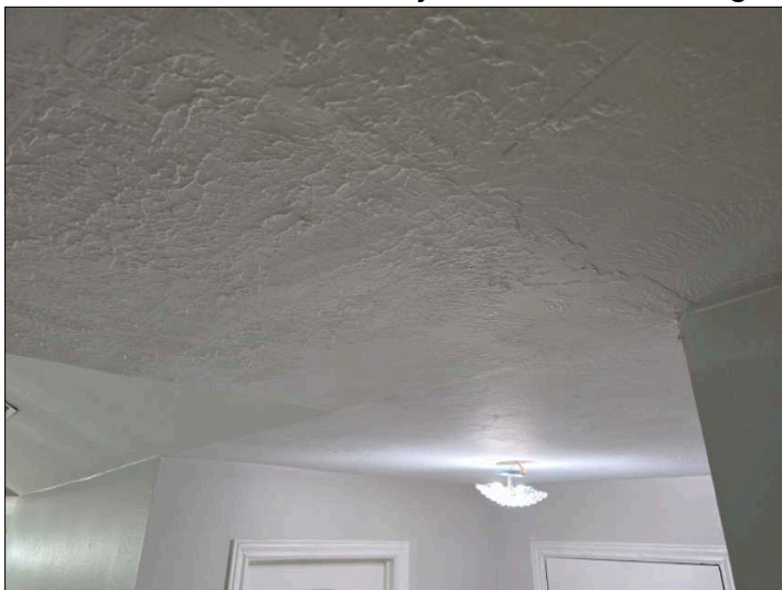
Ceiling is sagging. May be loose nails, or previous damage.
