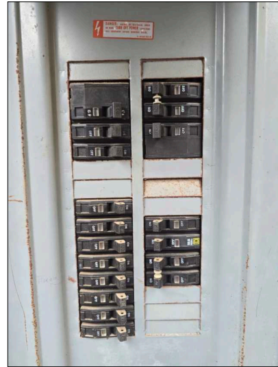
The electrical panel is not properly labeled.
