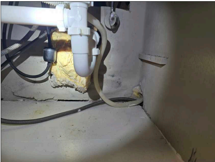
Active water leak in drain line of kitchen. Water pouring from exterior wall. Walls are likely heavily water and mold damaged. Full remediation suggested as needed.
