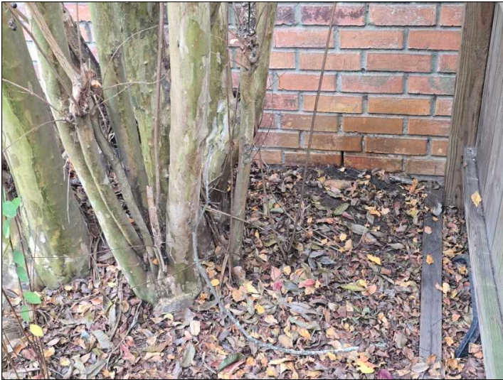
Tree root growth along house can be dangerous for roots in sewer lines, drainage, foundation issues and termites.
