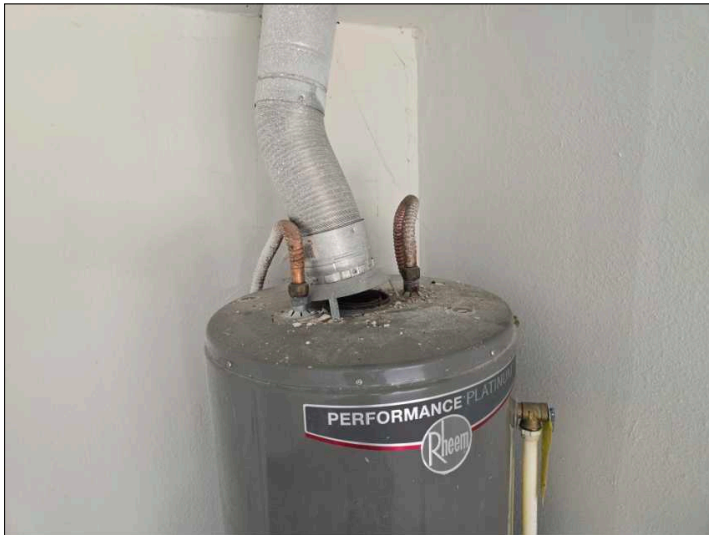
Flue pipe not secured to top of water heater. Heater exhaust gas leakage around flue catch. This should be repaired immediately.
