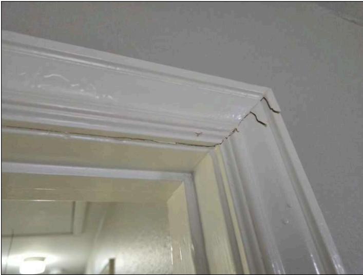
Shift settlement noted at door frame.
