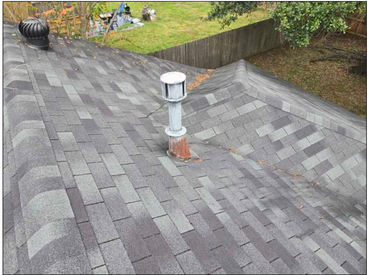
Rusted vents and flashing on roof.
