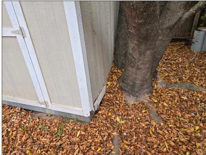
Shop too close to tree. Damage to side wall.
