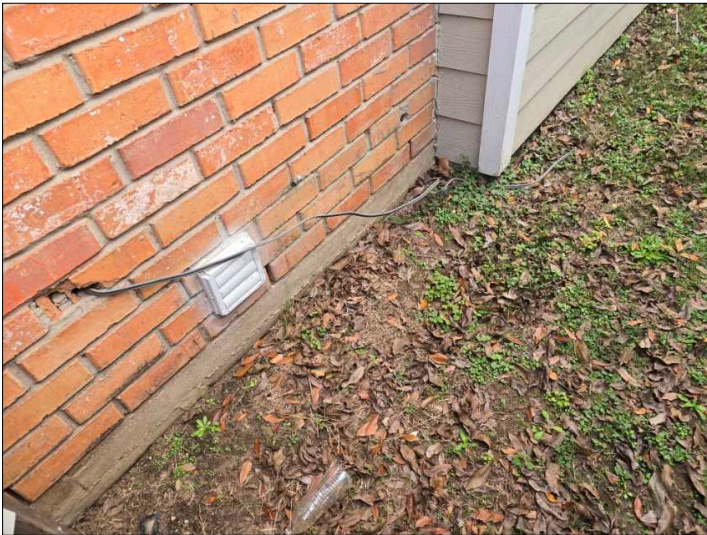
Dryer wire added to panel, but wire loosely exposed and not properly protected
