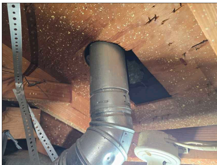
Flue should be clear of combustibles by minimum 1".
