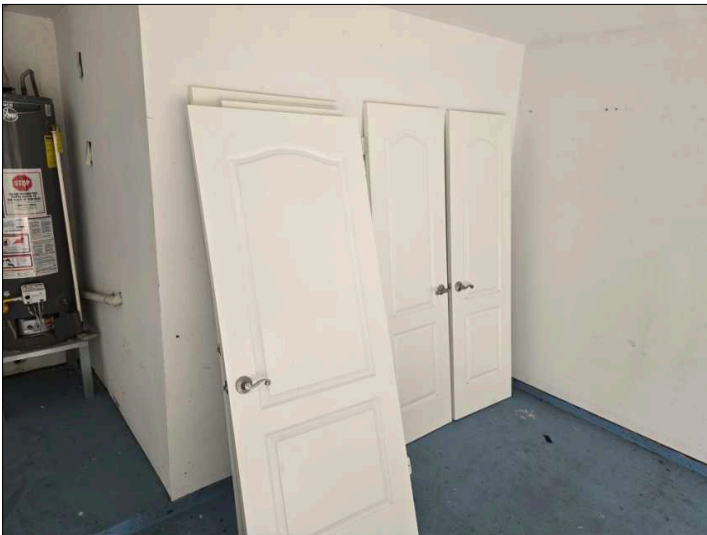
Many doors missing / not installed.
