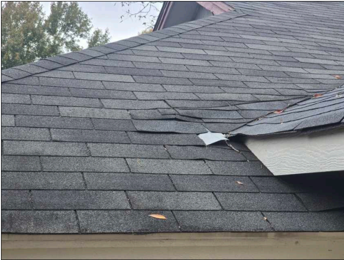
Evidence of previous repair. Multiple shingles present.
