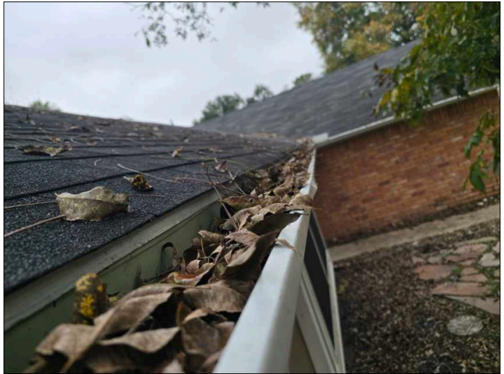
Heavy debris in gutters. These should be cleaned to provided good water flow away from house.
