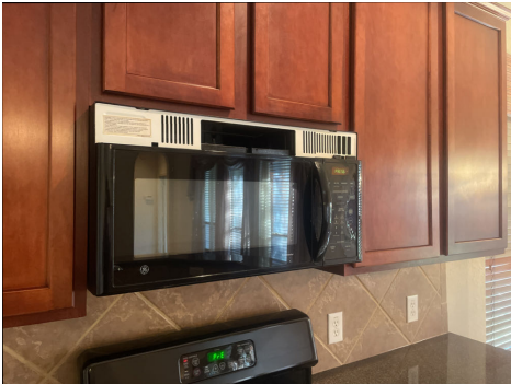
Vent cover missing.
