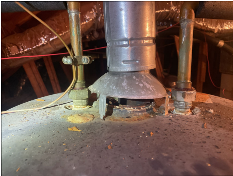
Draft hood needs adjustment
