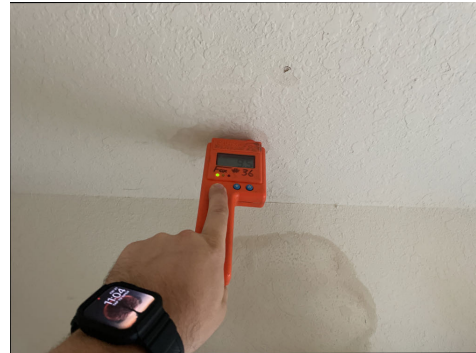
Stain dry at time of inspection
