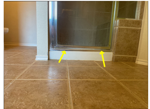
Missing weather stripping
