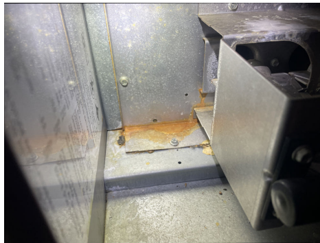
Rust stains in heater cabinet
