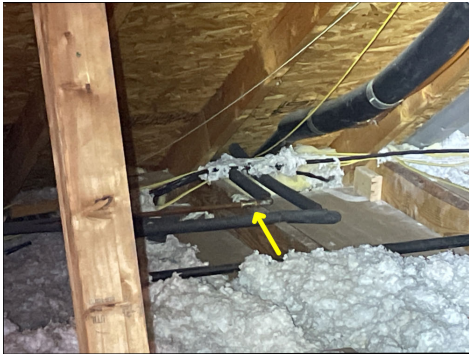
Evidence of a plumbing repair over the kitchen
