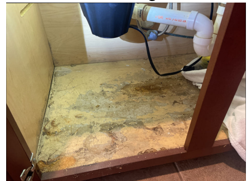
Water damage to cabinet base. Page 10 of 28
