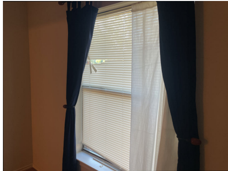
Window covering damaged.
