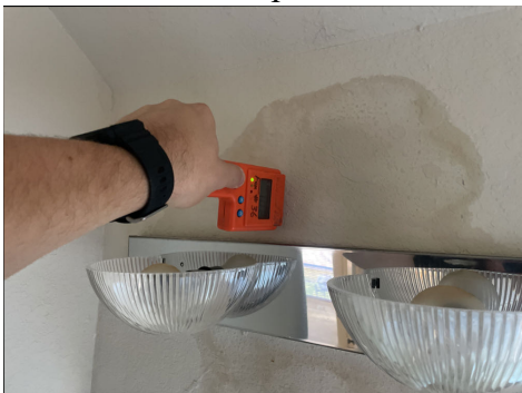
Stain dry at time of inspection REI 7-6 (8/9/21)
