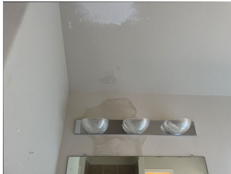
Stains dry at time of inspection
