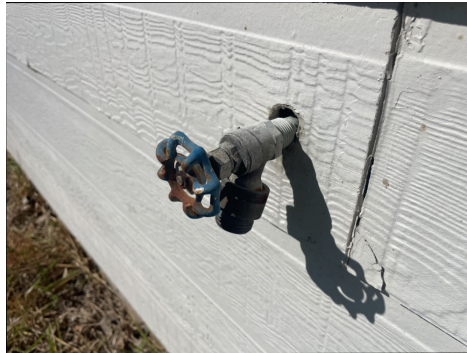
Hose bib missing finish ring.
