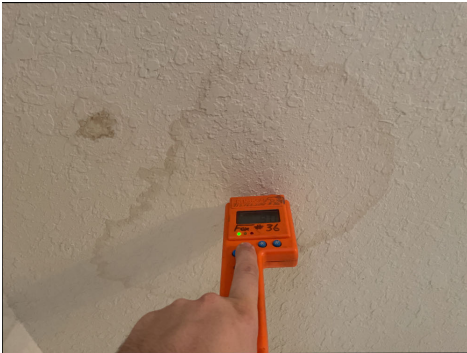
Stain dry at time of inspection
