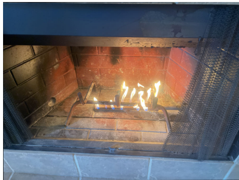
Fire place operational
