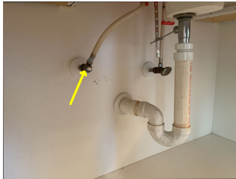
Missing shut off valve handle
