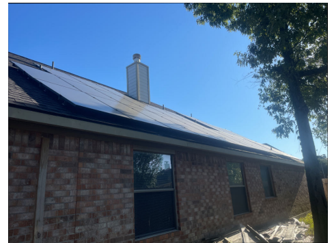
Proper installation of solar power system not checked.
