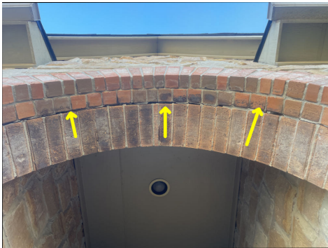
Cracks/ separation in brick work
