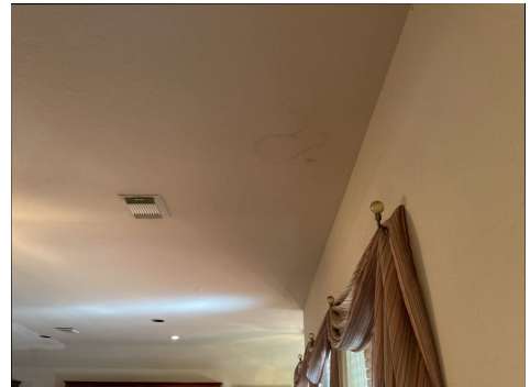
Stain dry at time of inspection
