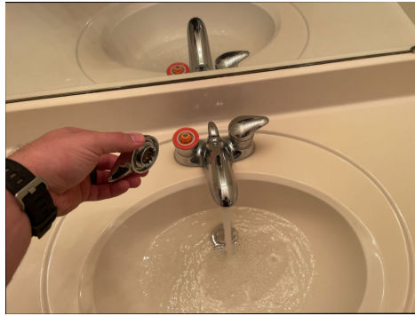
Faucet handle loose.
