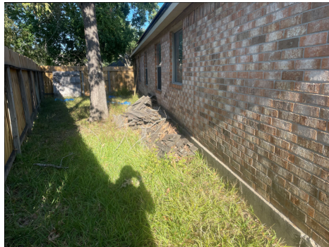
Stored wood near house should be moved
